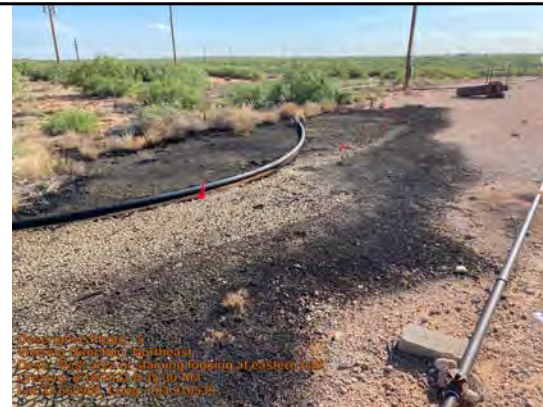
West area of staining looking at eastern half
