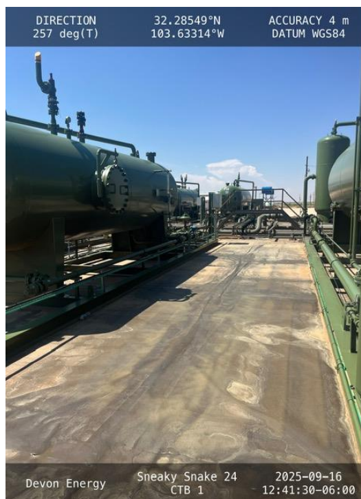
Photo 14 View of containment facing northwest.
