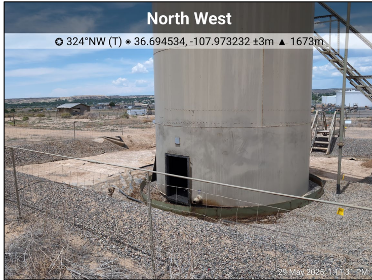
Photograph: 1 Date: 05/29/2025 Description: Soil staining in release footprint View: Northwest
