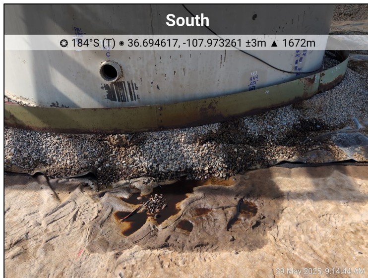
Photograph: 3 Date: 05/29/2025 Description: Soil staining at release point View: South
