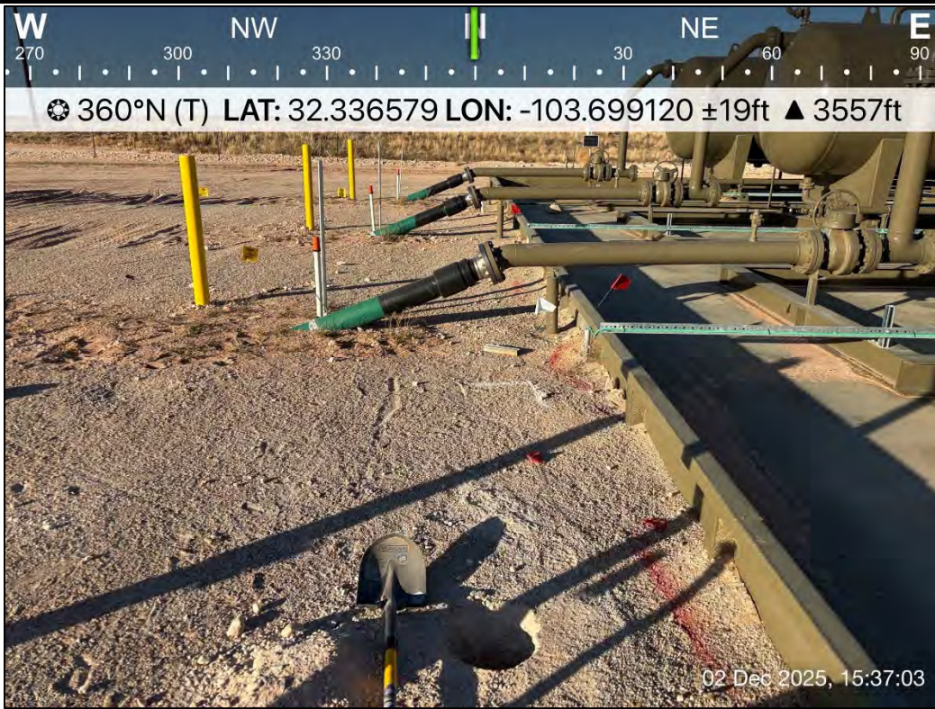
PHOTO 1: Northern view during additional delineation activities. 12/02/2025
