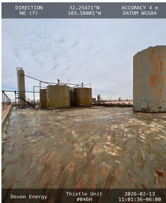
Photo 3 View of south side of secondary containment towards northeast. Residual moisture from recent rainfall event.
