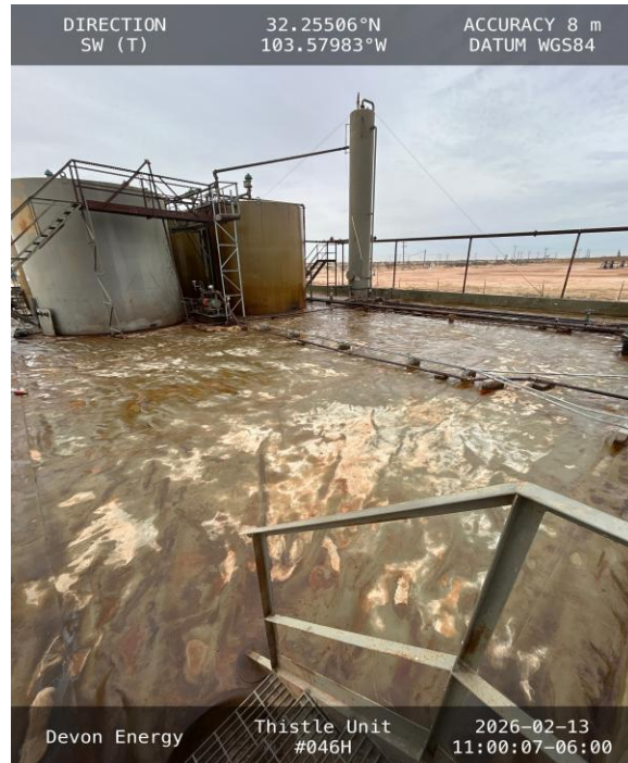
Photo 2 View of north side of secondary containment towards southwest. Residual moisture from recent rainfall event.
