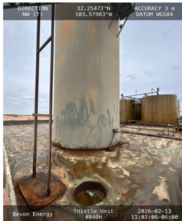
Photo 4 View of south side of secondary containment towards northwest. Residual moisture from recent rainfall event.
