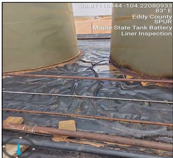
Photo taken pursuant to power washing. Facing east.
