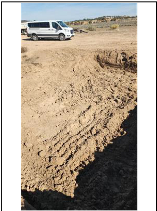
Photo 6 Final excavation. Looking northeast with view of base, north and east wall.
