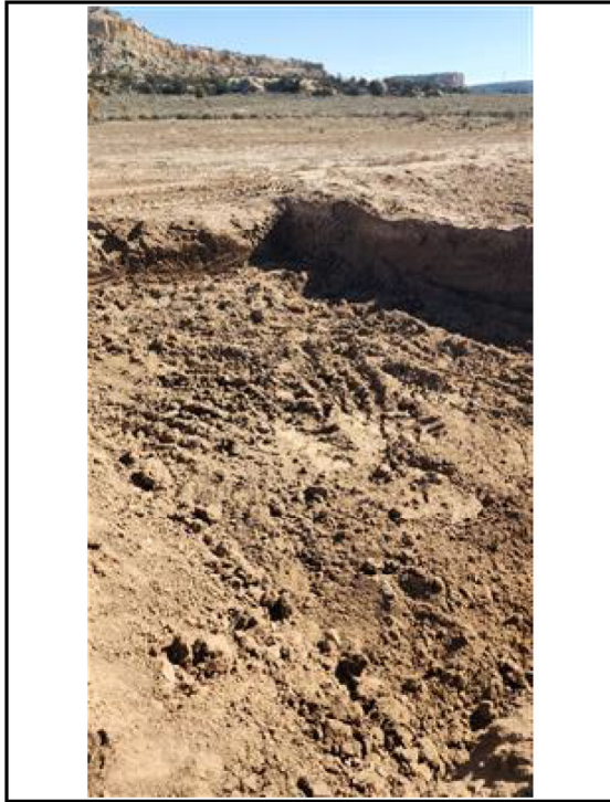
Photo 4 Final Excavation. Looking southeast with view of base, south and east wall.
