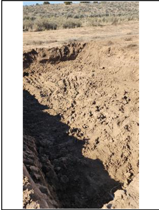
Photo 8 Final Excavation. Looking northwest with view of base, north and west wall.
