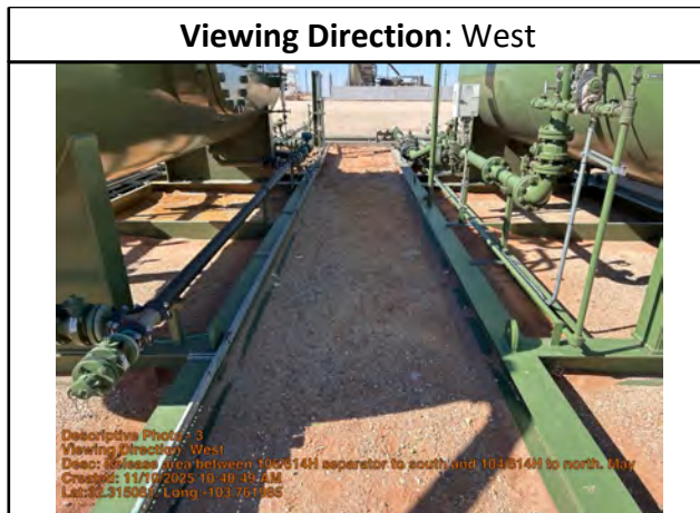
Release area between 106/614H separator to south and 104/814H to north. May need to advance north delineation point north of 104/814H separator.
