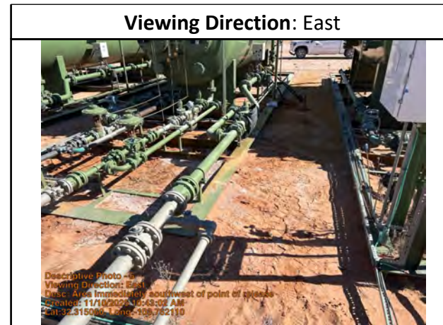
Area immediately southwest of point of release. BH25-01 between 614H and 703H for vertical delineation.
