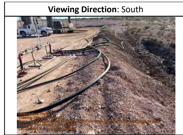
West edge of pad facing south. Poly lines over berm off west edge of pad.
