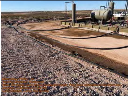
On slope south of pad facing northwest. Poly lines between containment and edge of pad.
