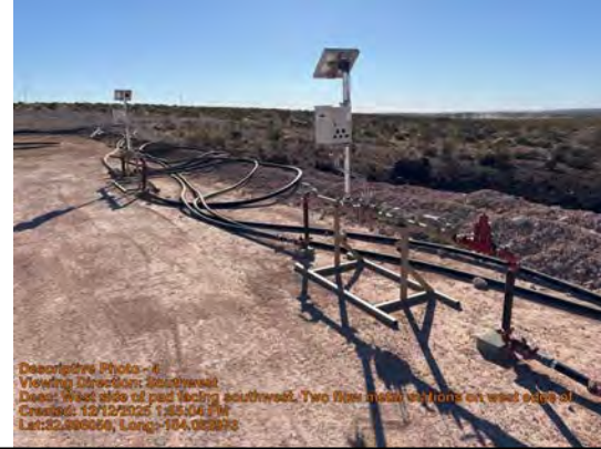
West side of pad facing southwest. Two flow meter stations on west edge of pad.
