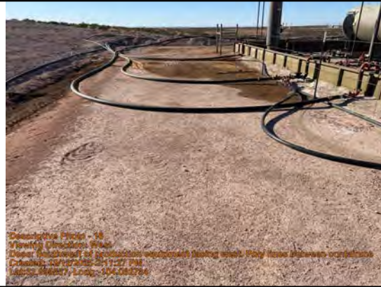
Southwest of production equipment facing west. Poly lines between containment and edge of pad.
