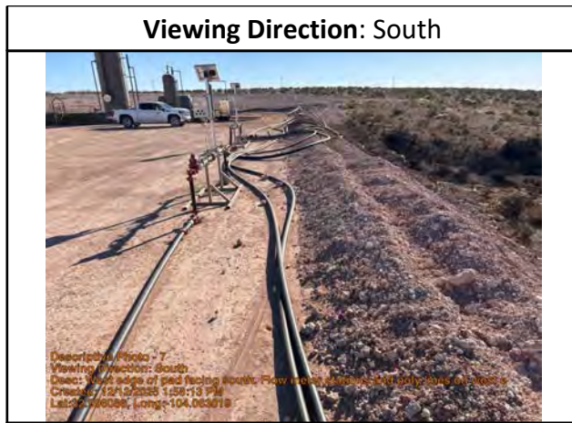
West edge of pad facing south. Flow meter stations and poly lines on west edge of pad.
