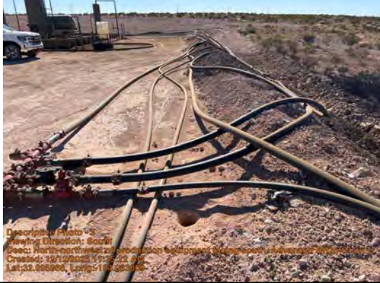
North-northwest of production equipment facing south. Advanced BH25-64 on west edge of pad.
