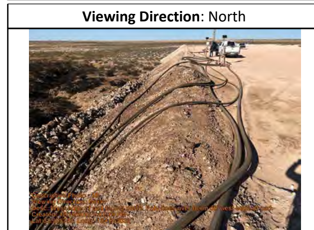
West edge of pad facing north. Poly lines over berm off west edge of pad.
