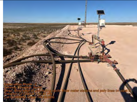
West edge of pad facing north. Flow meter stations and poly lines on west edge of pad.
