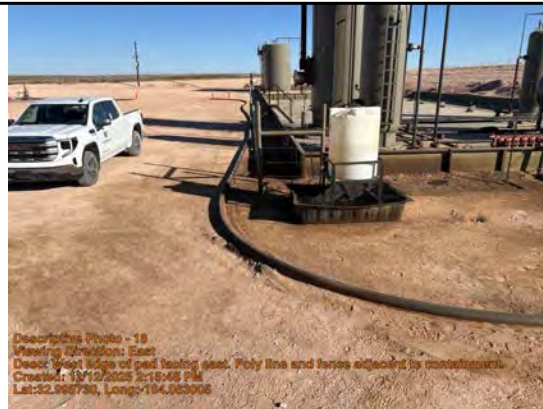
West edge of pad facing east. Poly line and fence adjacent to containment.
