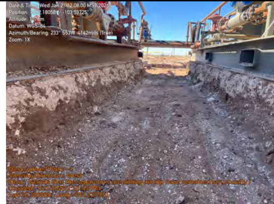
Islands that the separators are sitting on top have remained structurally intact.
