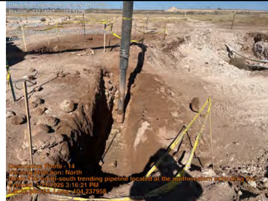
The north-south trending pipeline located at the northwestern extending the pad is being hydrovac to step out WS25-20 at 0-4ft.
