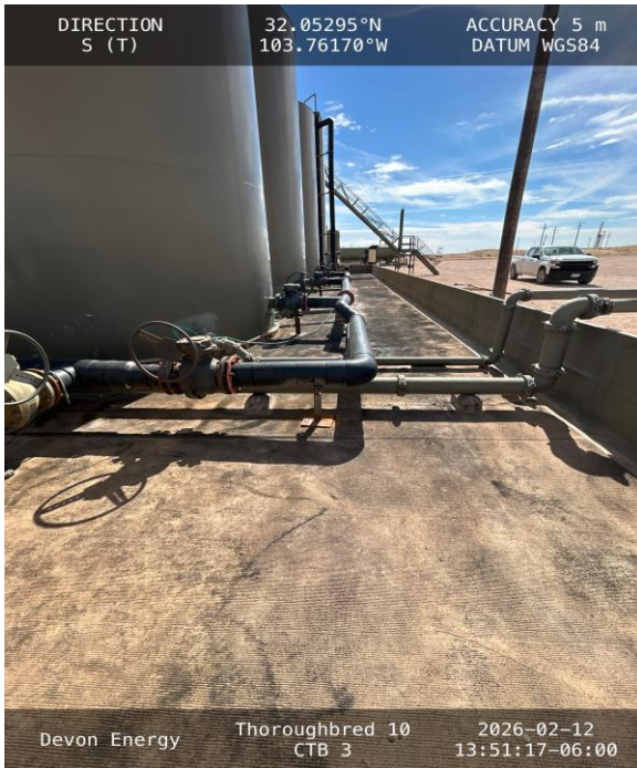
Photo 11 View of west side of secondary containment towards south.
