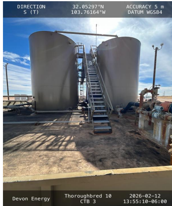
Photo 2 View of central portion of secondary containment.
