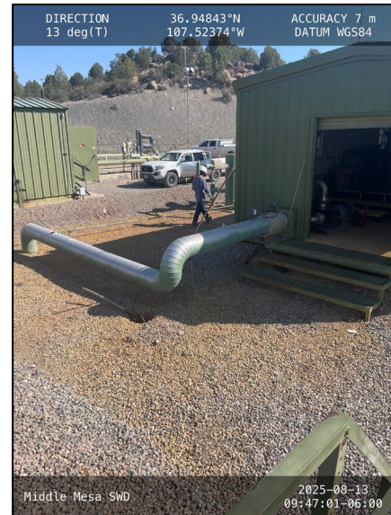
Photograph: 2 Date: 8/13/2025 Description: Location HA01/PH01 and area just outside equipment building View: North
