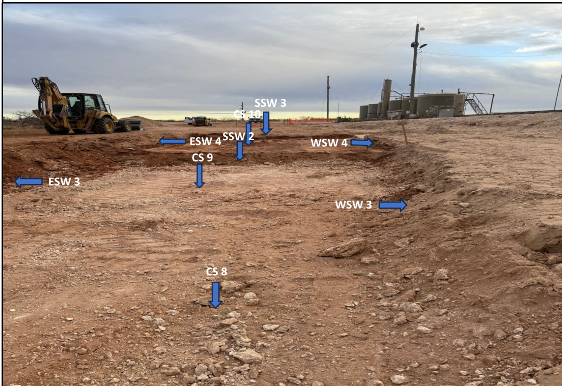
View South - Remediation activities (i.e., excavation and stockpiling) in progress. Sample locations CS 8 thru CS 10, ESW 3, ESW 4, SSW 2, SSW 3, WSW 3, and WSW 4.
