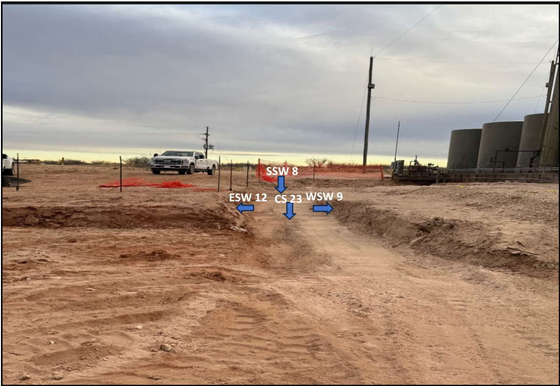
View South - Remediation activities (i.e., excavation and stockpiling) in progress. Sample locations CS 23, WSW 9, ESW 12, and SSW 8.
