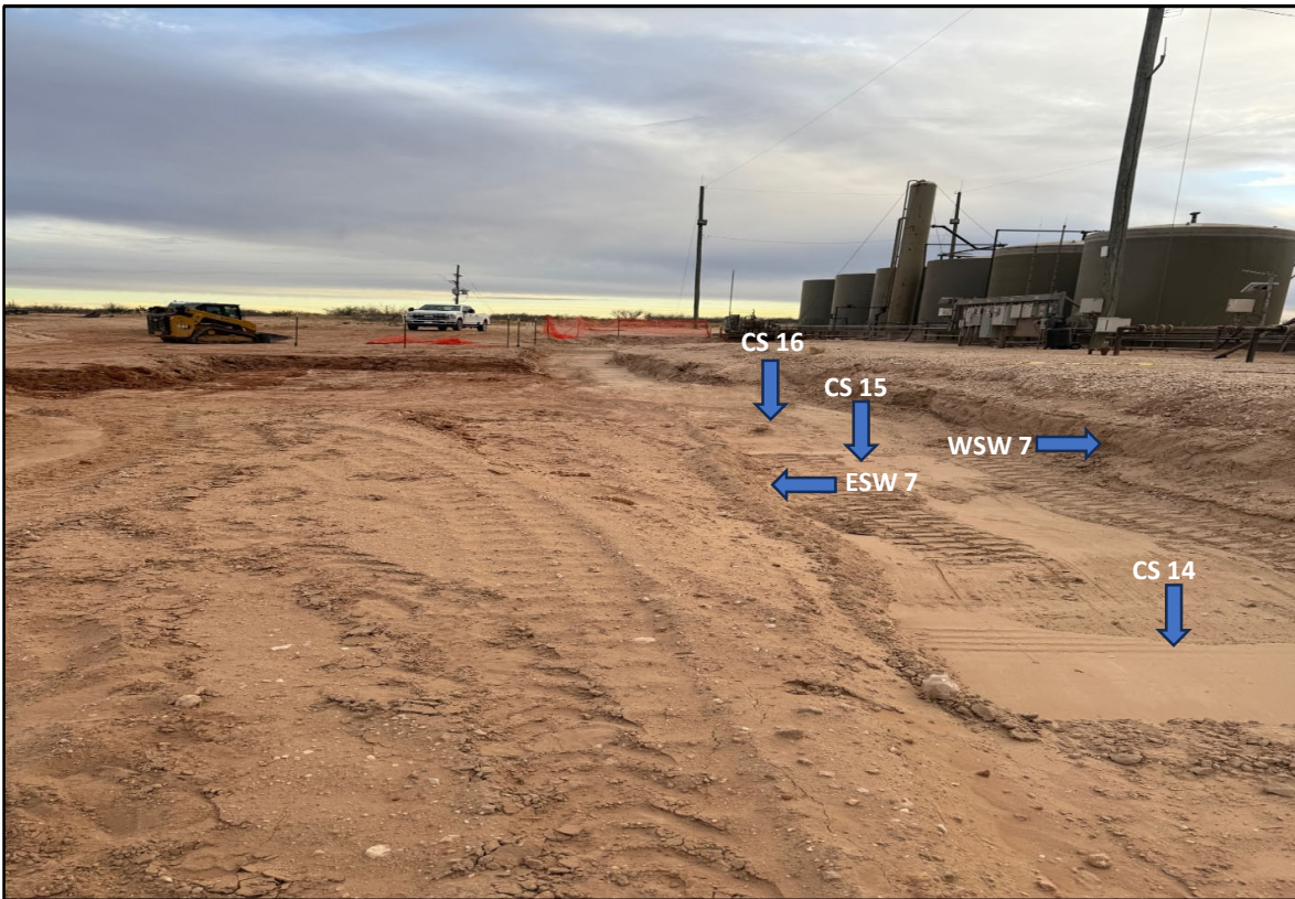
View South - Remediation activities (i.e., excavation and stockpiling) in progress. Sample locations CS 14 thru CS 16, WSW 7, and ESW 7.
