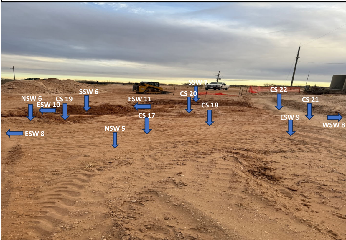
View South - Remediation activities (i.e., excavation and stockpiling) in progress. Sample locations CS 17 thru CS 22, NSW 5, NSW 6, WSW 8, ESW 8 thru ESW11, SSW 6, and SSW 7.
