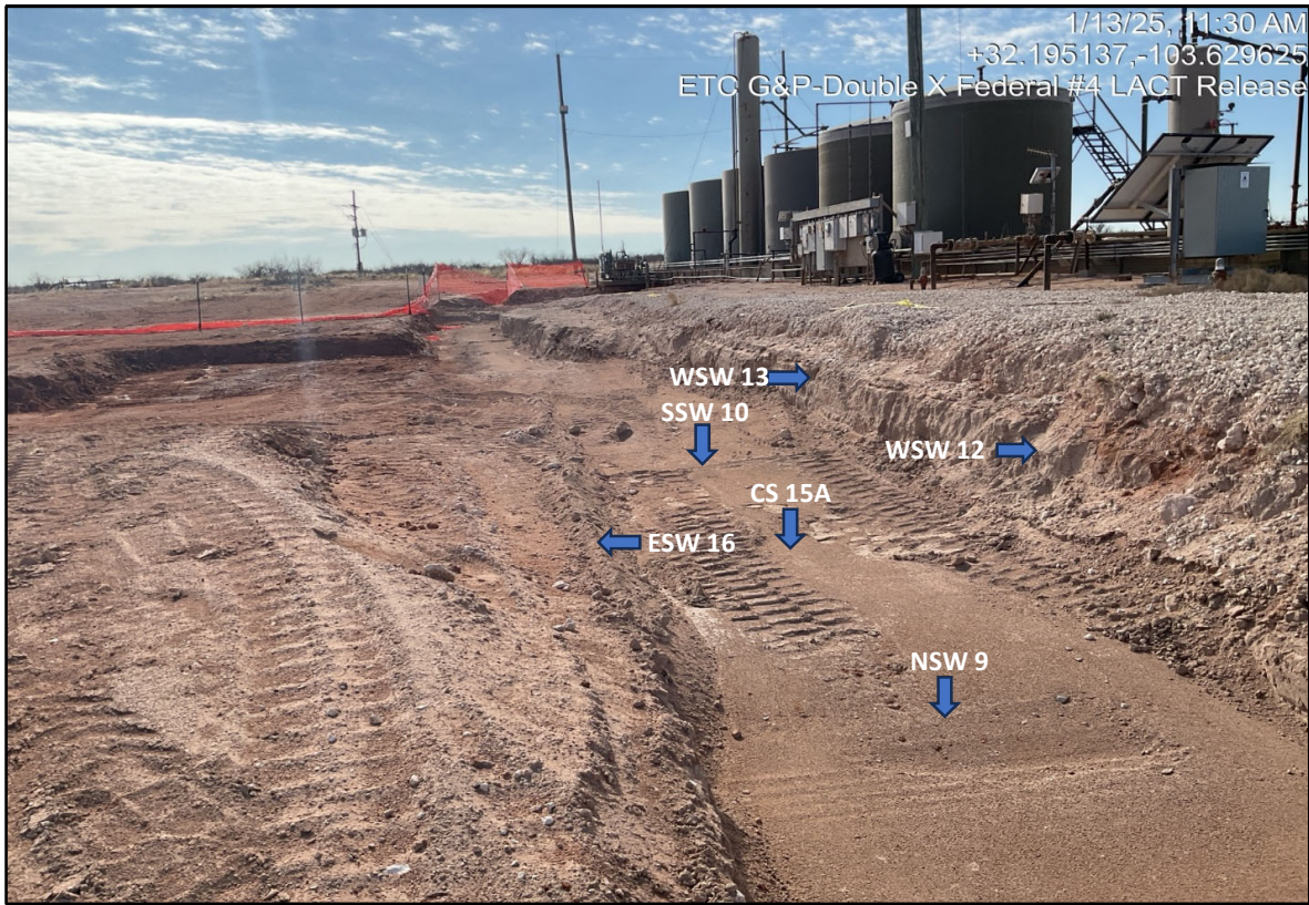
View South - Remediation activities (i.e., excavation and stockpiling) in progress. Sample locations CS 15A, NSW 9, WSW 12, WSW 13, ESW 16, and SSW 10. Date: Jan 13, 2025
