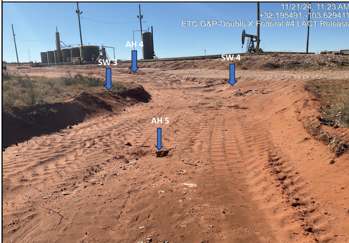
View North - Remediation activities (i.e., excavation and stockpiling) in progress. Sample locations AH 4, AH 5, SW 3, and SW 4.
