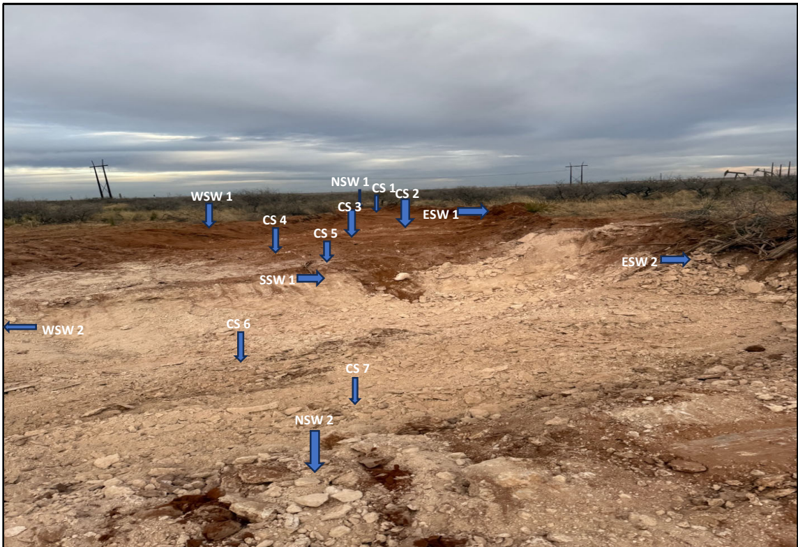
View East - Remediation activities (i.e., excavation and stockpiling) in progress. Sample locations CS 1 thru CS 7, NSW 1, NSW 2, ESW 1, ESW 2, SSW 1, WSW 1, and WSW 2.
