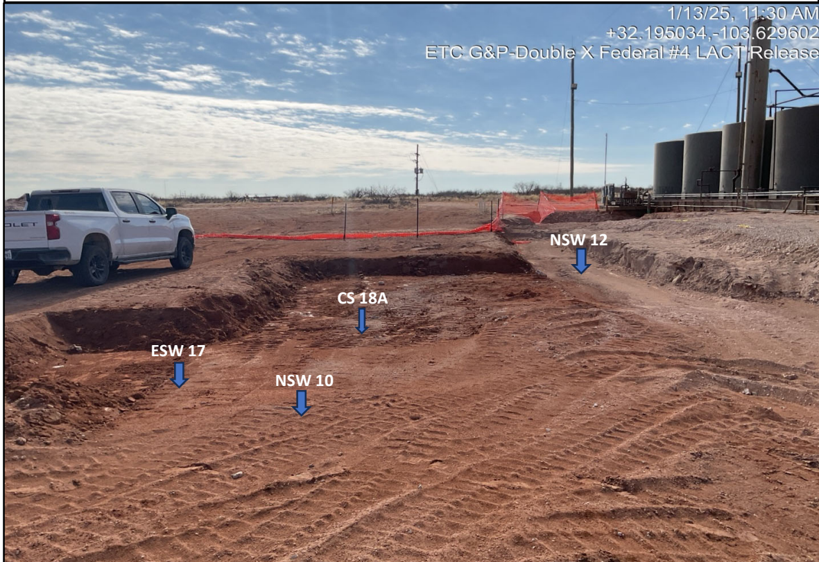
View South - Remediation activities (i.e., excavation and stockpiling) in progress. Sample locations CS 18A, NSW 10, NSW 12, and ESW 17. Date: Jan 13, 2025
