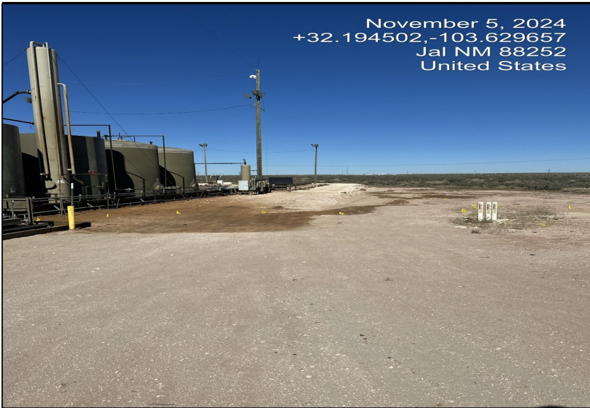
View North - A portion of the release footprint. Note the surface staining (i.e., dark brown color). Release caused by a corroded valve on a LACT unit. Date: Nov 05, 2024
