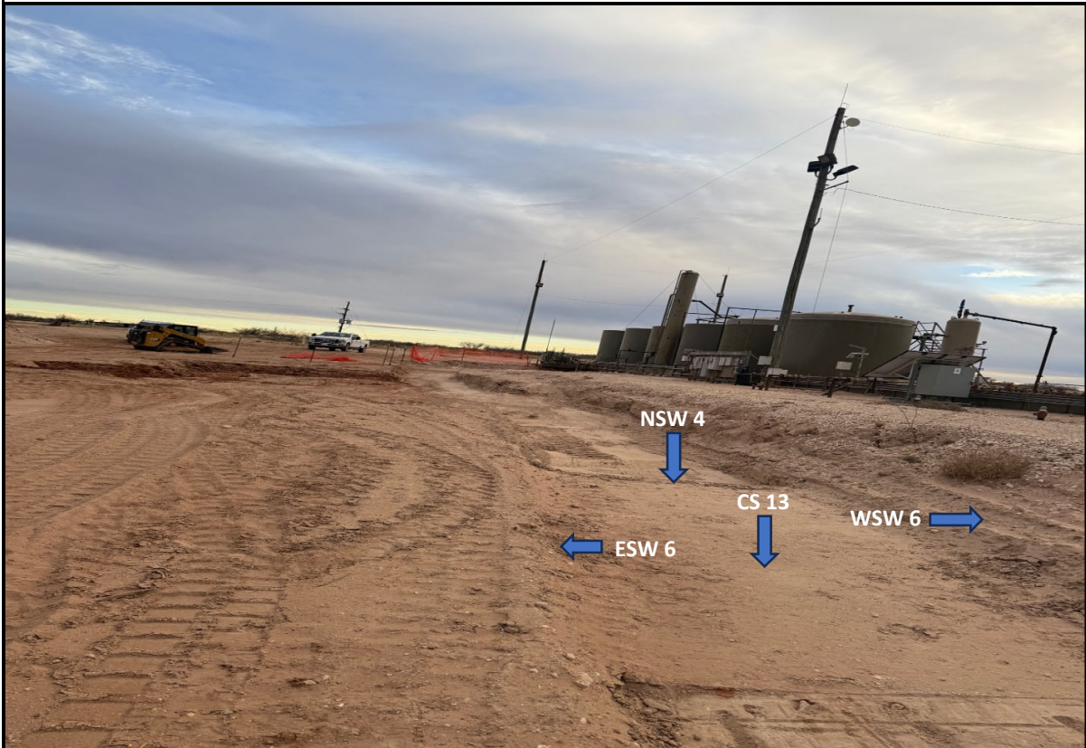
View South - Remediation activities (i.e., excavation and stockpiling) in progress. Sample locations CS 13, NSW 4, WSW 6, and ESW 6.
