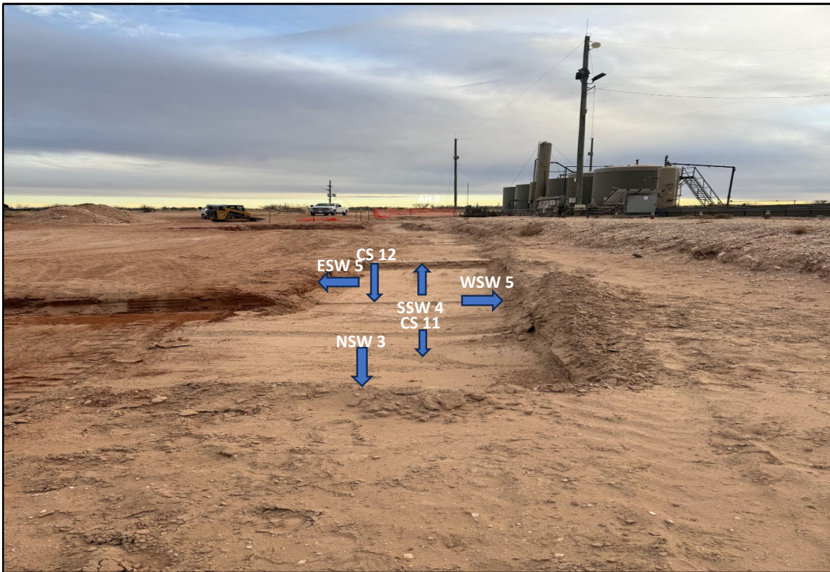
View South - Remediation activities (i.e., excavation and stockpiling) in progress. Sample locations CS 11, CS 12, NSW 3, WSW 5, ESW 5, and SSW 4.
