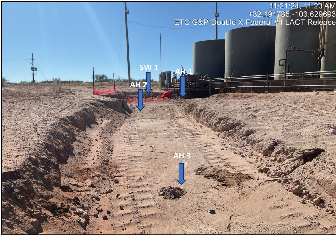
View South - Remediation activities (i.e., excavation and stockpiling) in progress. Sample locations AH 1 thru AH 3 and SW 1.
