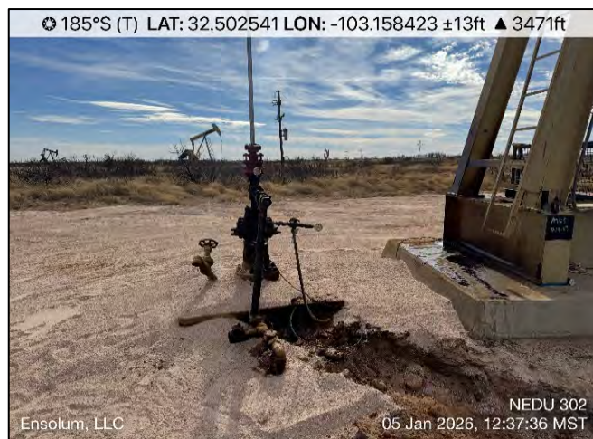
Photograph: 1 Date: 1/5/2026 Description: Soil staining near wellhead View: South
