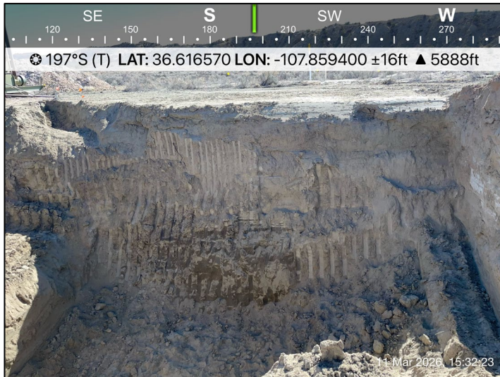
Photograph: 9 Description: Staining on south sidewall View: South Date: 3/11/2026
