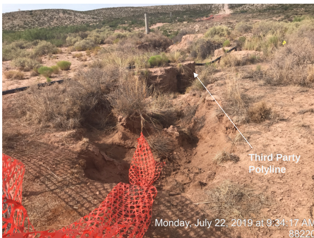
East side of the river, looking west washout
