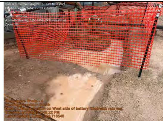
2' excavation on West side of battery filled with rain water
