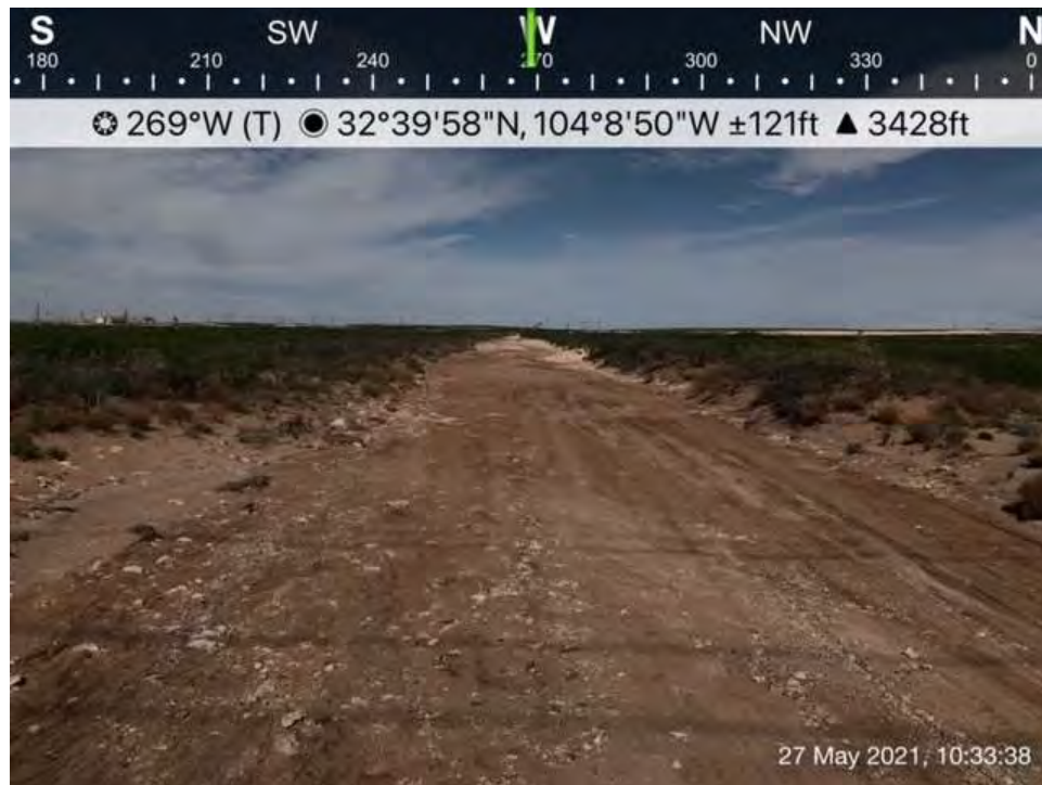
Saturated soil on lease road, Spill Area C, viewing to the west.
