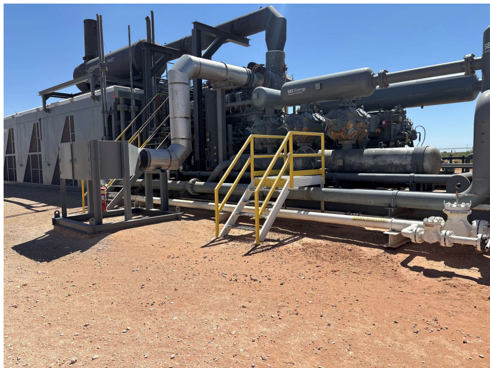
Photo 6 View of Unit 2707 compressor skid at Alamo Compressor Station
