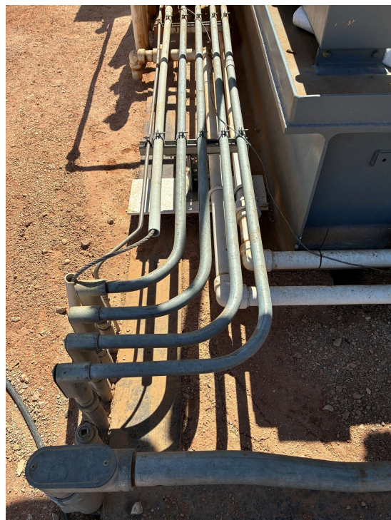
Photo 12 View of Unit 2707 compressor skid at Alamo Compressor Station
