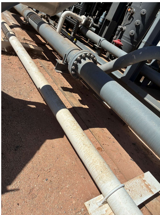
Photo 13 View of Unit 2707 compressor skid at Alamo Compressor Station
