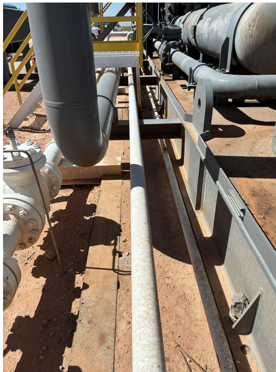
Photo 10 View of Unit 2707 compressor skid at Alamo Compressor Station
