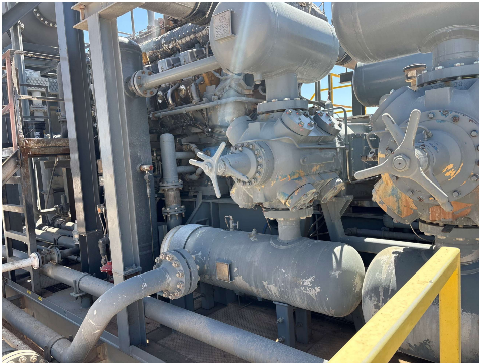
Photo 9 View of Unit 2707 compressor skid at Alamo Compressor Station
