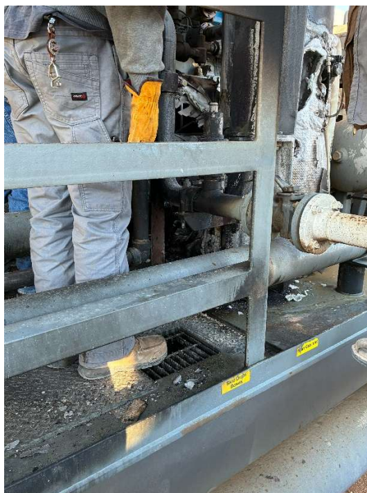
Photo 2 View of affected area confirming no release of fluids to surrounding area.
