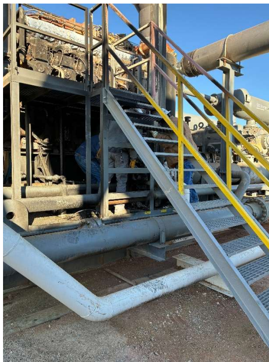
Photo 1 View of affected skid area and adjacent pad area prior to repairs.
