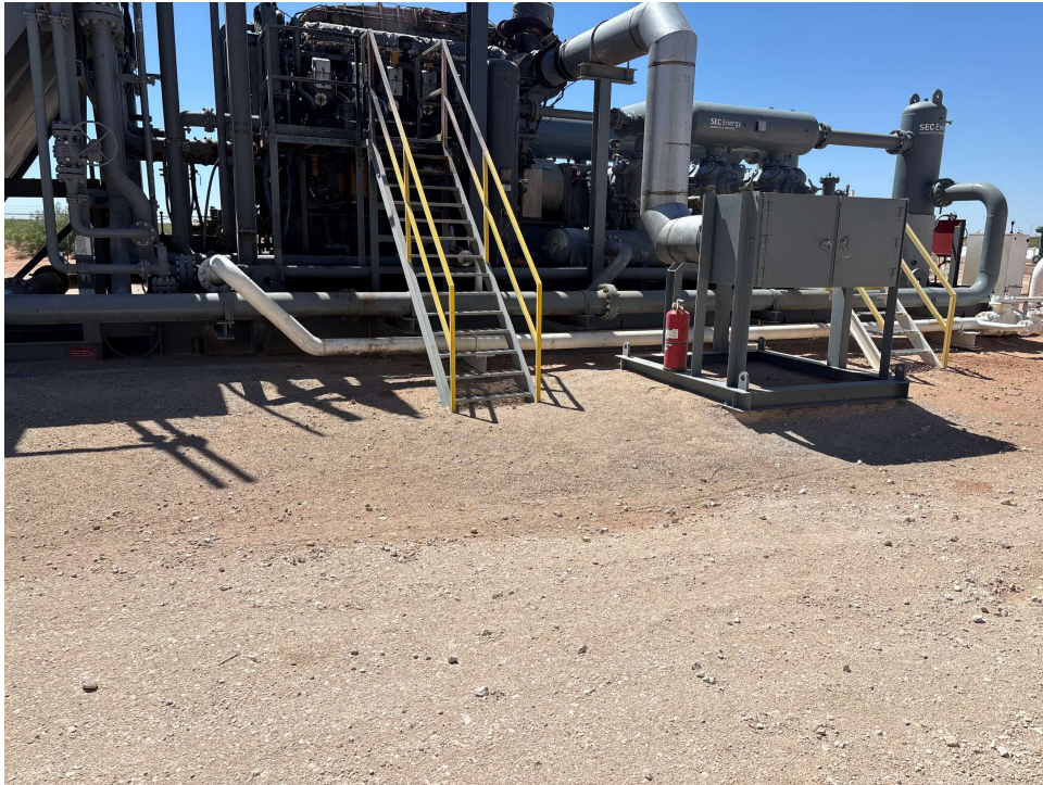
Photo 5 View of Unit 2707 compressor skid at Alamo Compressor Station
