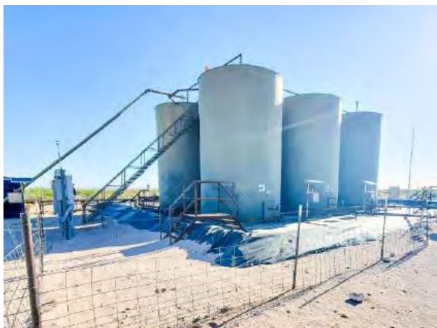
Photograph 9: View of tank battery and liner
