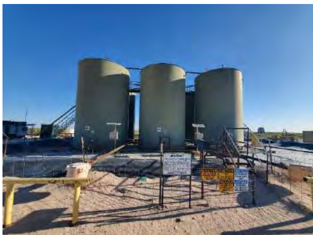
Photograph 8: View of tank battery and liner
