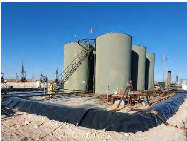
Photograph 7: View of tank battery and liner
