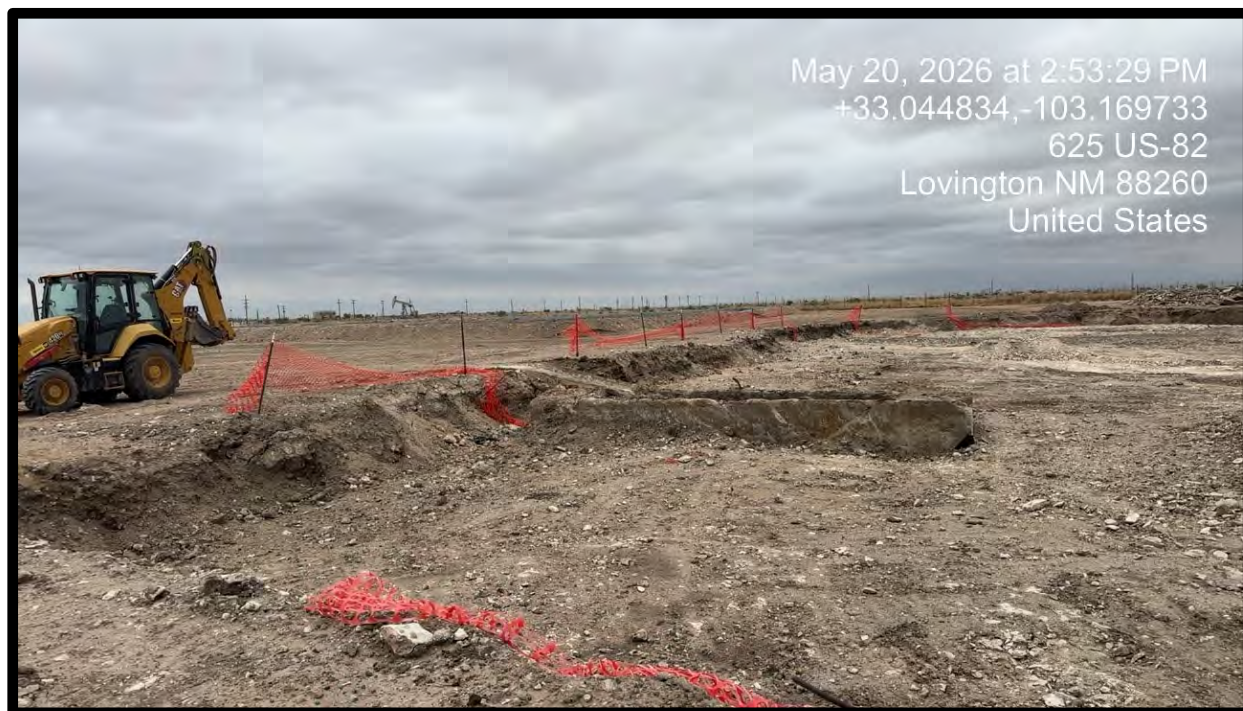
PHOTOGRAPH NO. 4 – An area of remnant cement with no soil available for sampling. DGP requests that these areas be exempt from the sampling process. The view is towards the northwest.
