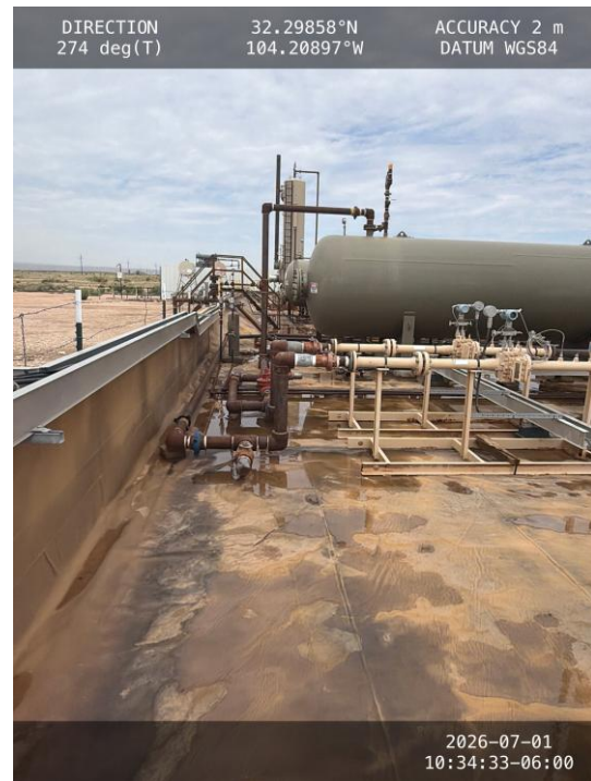
Photo 2 View of the containment area facing west. Residual water from rainfall event.
