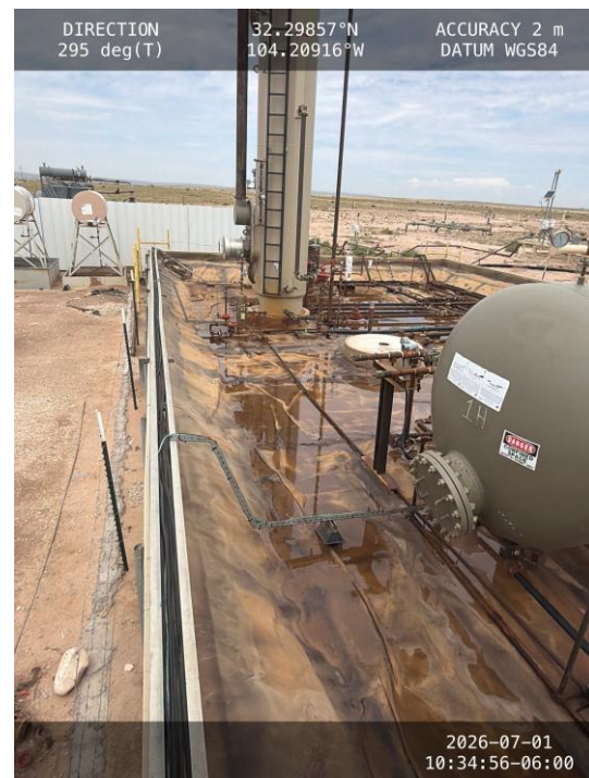
Photo 2 View of the liner corner of the containment area facing west northwest. Residual water from rainfall event.
