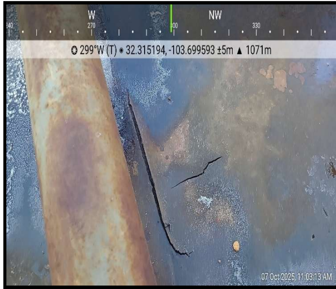
View of Liner Crack
