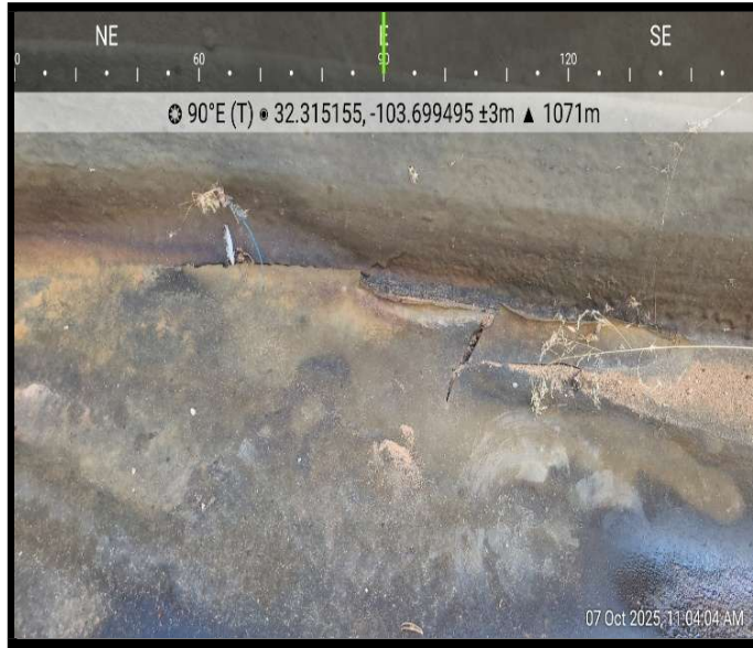
View of Liner Crack
