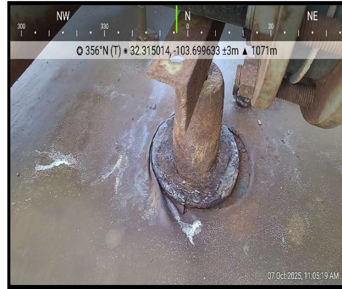
View of Liner Crack
