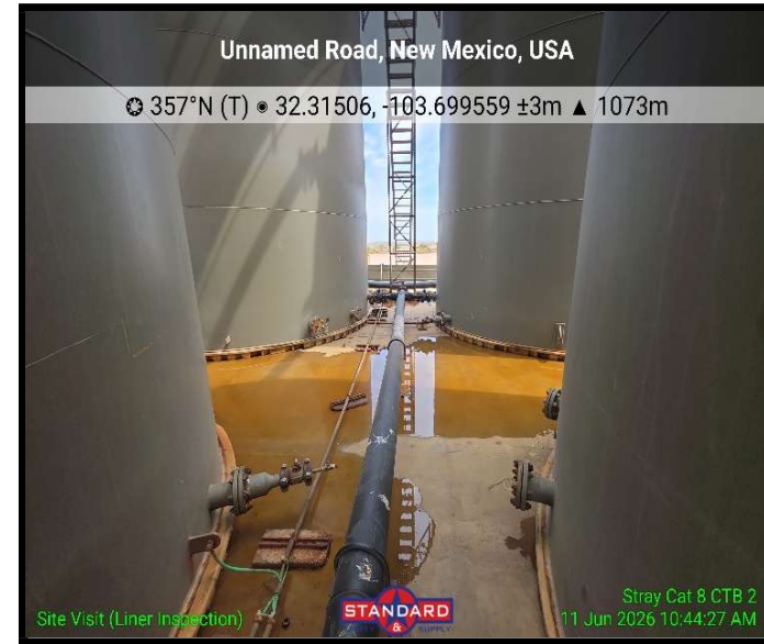
View of fluid in Secondary Containment
