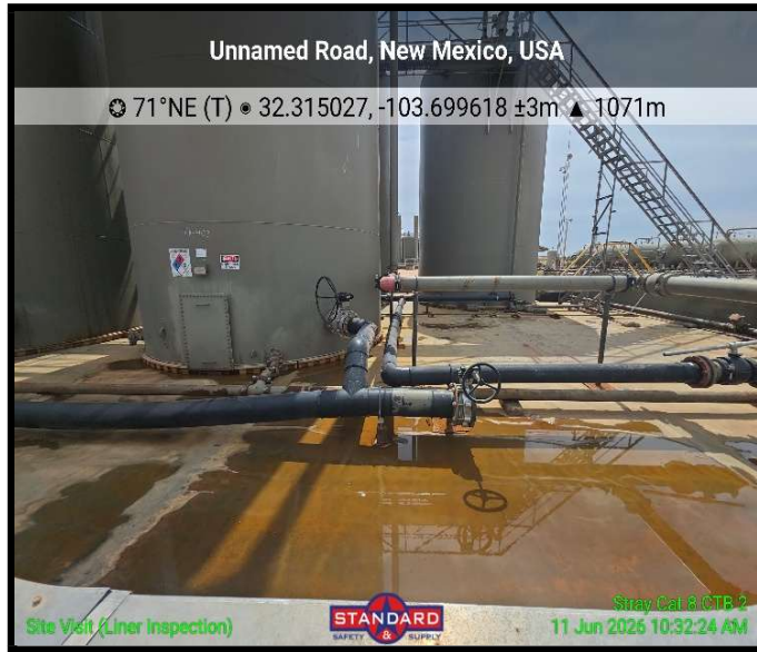
View of fluid in Secondary Containment
