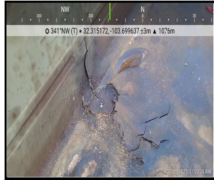
View of Liner Crack
