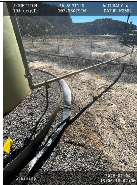
Photograph: 2 Date: 02/04/2026 Description: Soil staining within release footprint
