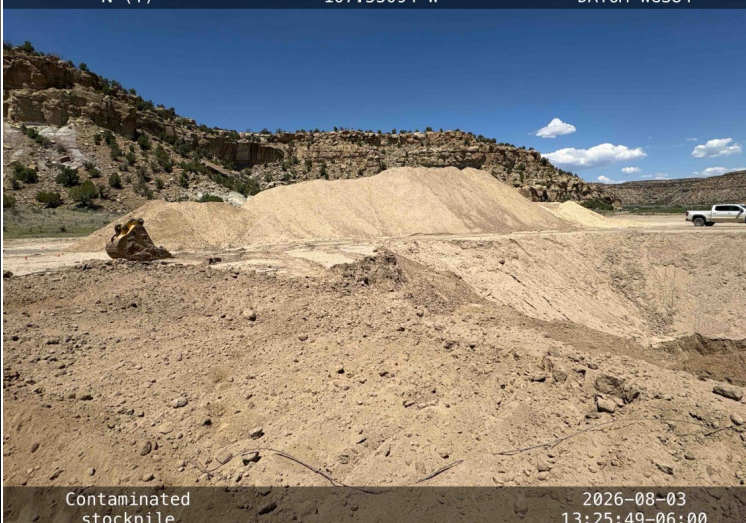
Photograph: 8 Date: 8/03/2026 Description: Contaminated stockpile north of excavation View: North
