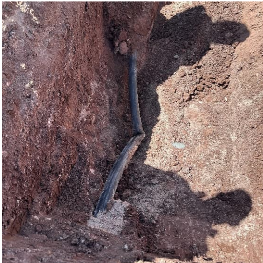
Photo 3. Groundwater Extraction System Piping
