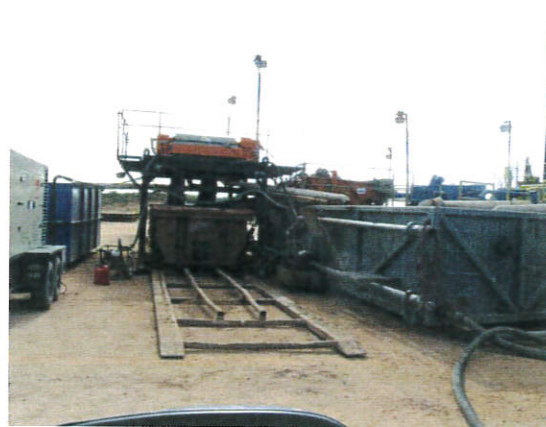
Above: Centrifugal Closed Loop System
