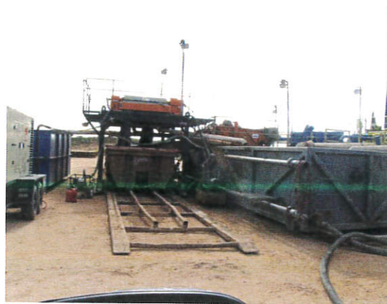
Above: Centrifugal Closed Loop System
