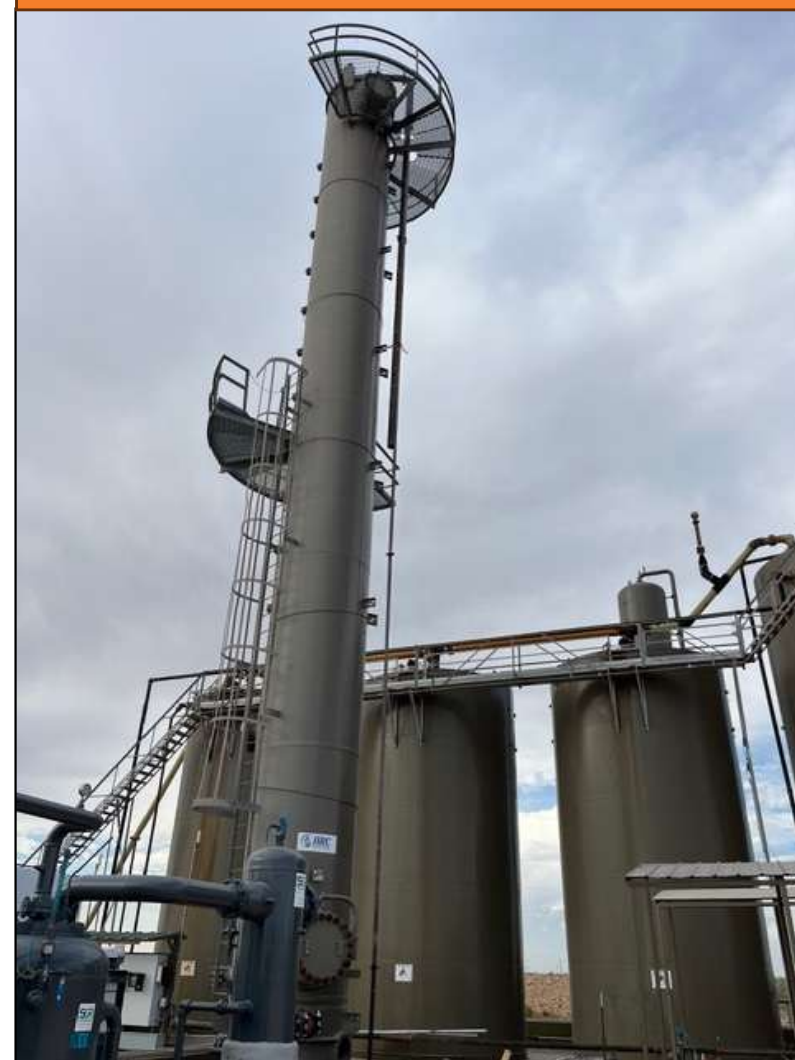
Oil H 2 S Treatment – Contact Tower
