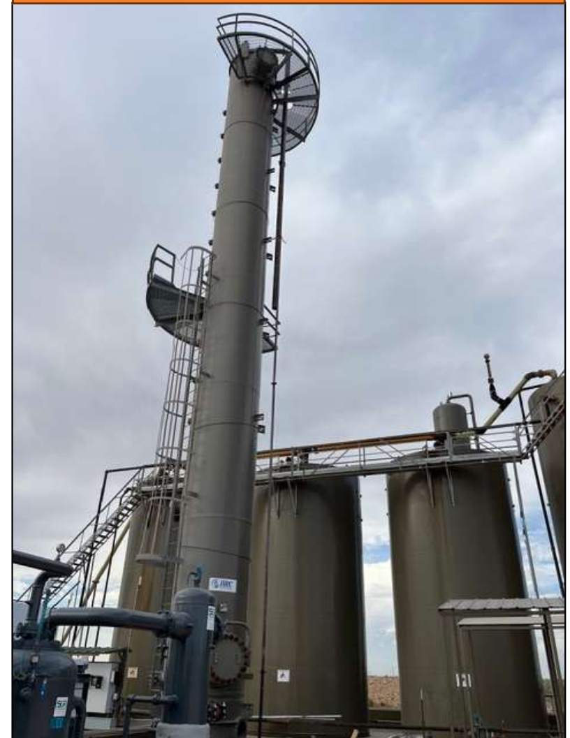
Oil H 2 S Treatment – Contact Tower
