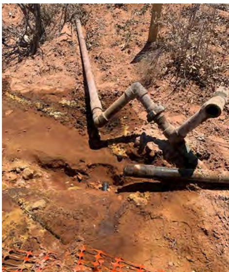
Photograph 1: Source of release (2" flow line)
