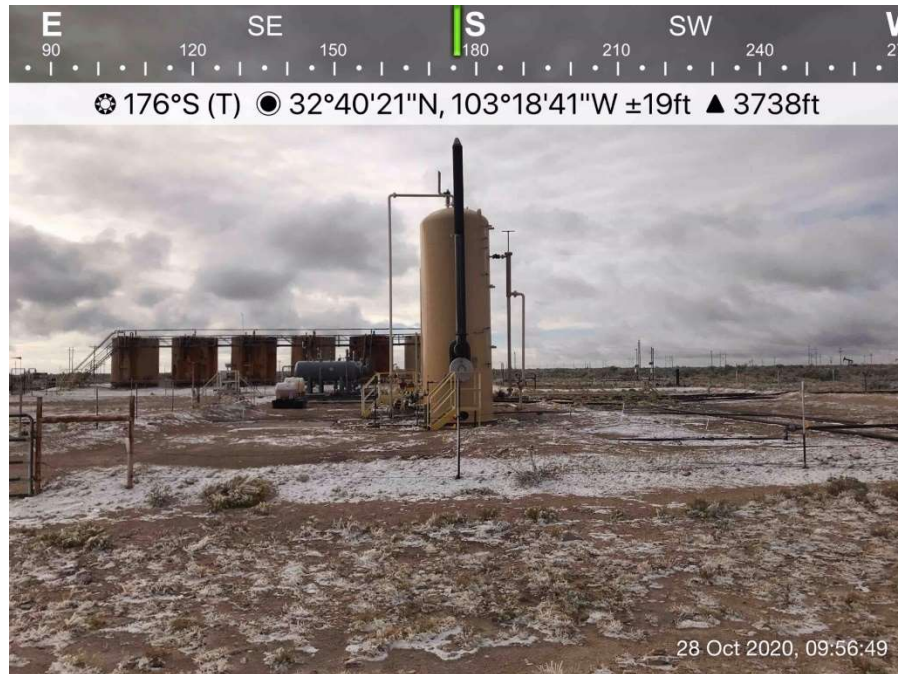
Impacted area viewing south, October 28, 2020
