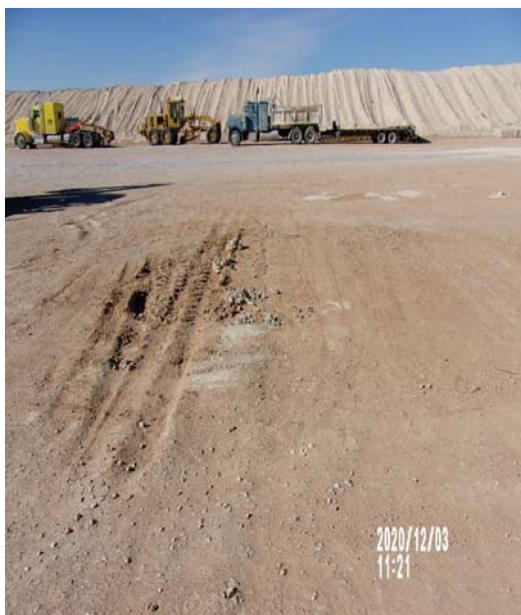
View West – Origin of spill. Release caused by open frac tank valves and a failed liner at an adjacent containment.
