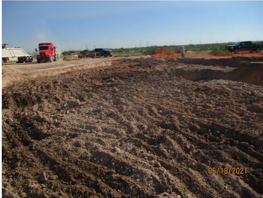
Typical view of excavated area as it neared completion. Shallow Excavation Area 4 pictured in foreground.
