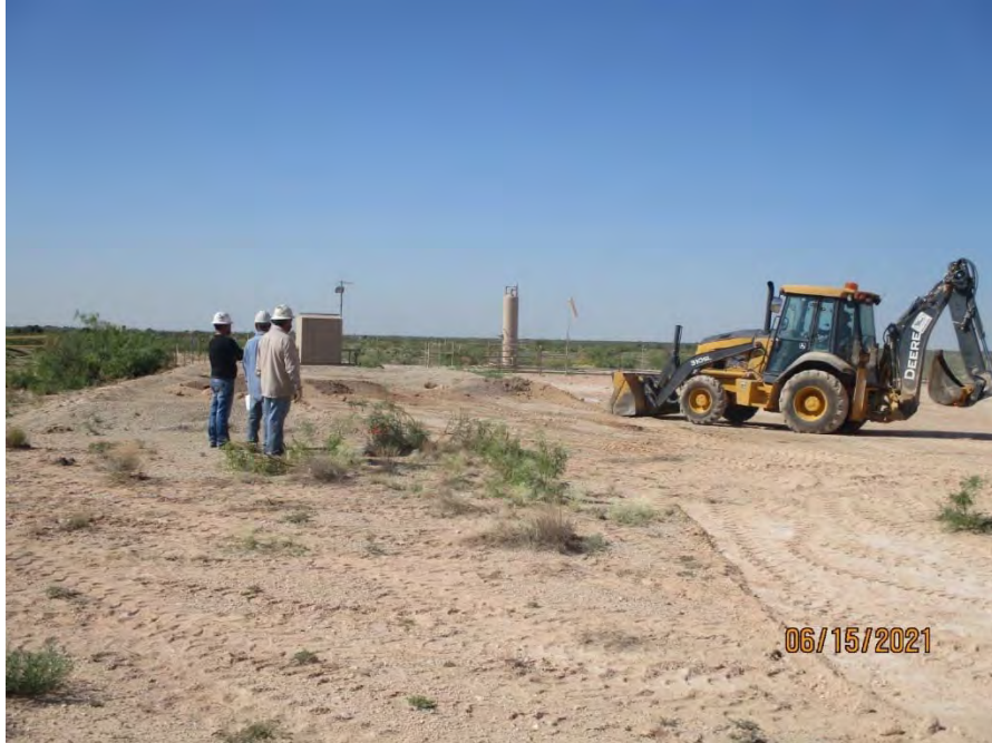
View of the tank battery area on June 15, 2021, following removal of the tanks. Contractor is removing the pea gravel/caliche from the former tank battery for off-site disposal.
