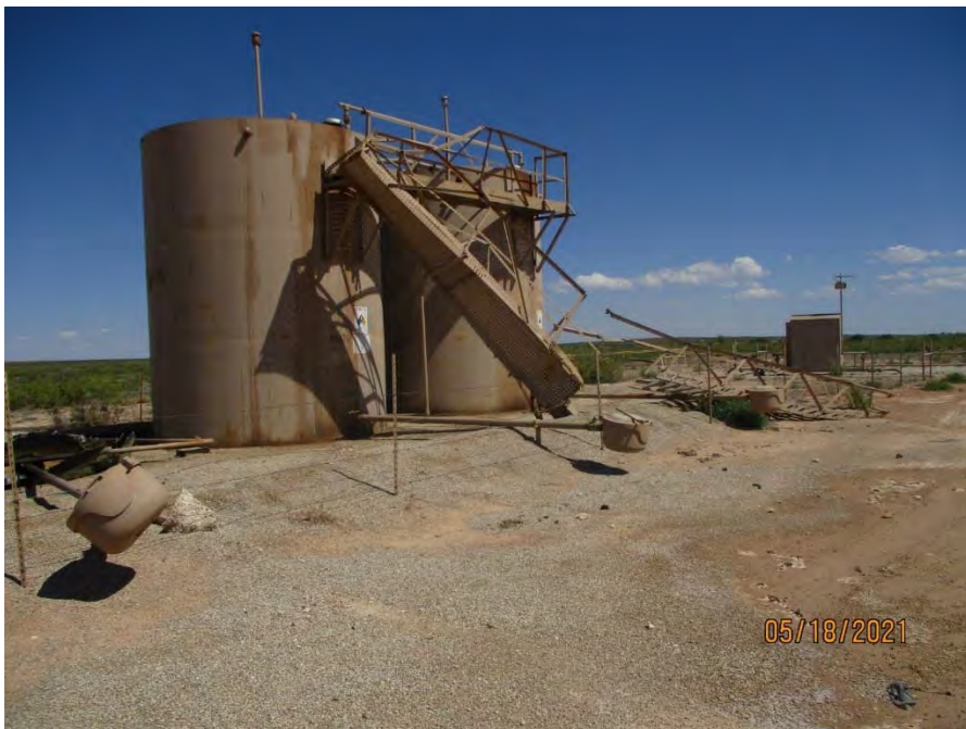
Another view of the lightning-damaged tank battery taken during the initial Ranger site inspection on May 18, 2021. View towards the southeast.
