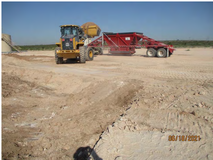
Typical view of trucks being loaded with excavated soil for off-site disposal.
