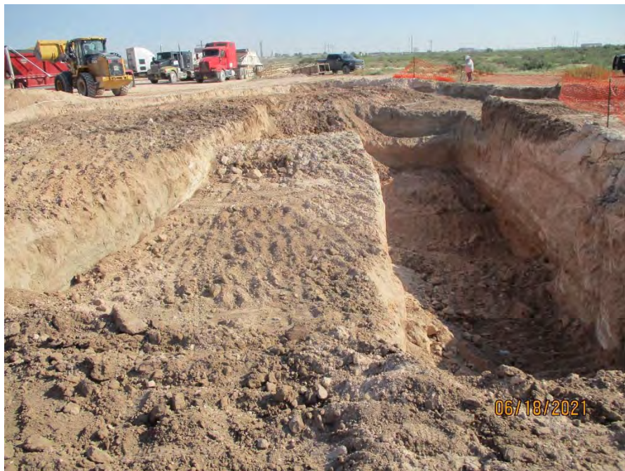
View of Excavation Area 5 (on left, ~3'-5' deep) and Excavation Area 3 (on right, ~12'-13' deep)
