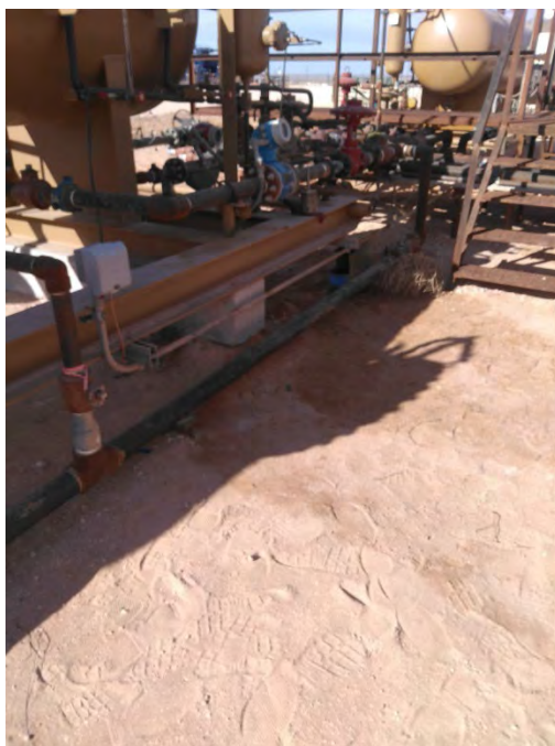
Photo 6: Northeast view visibly affected soil under process piping and equipment.
