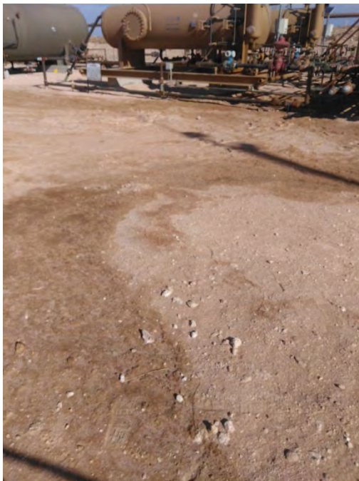
Photo 5: Northwest view of visibly affected area under process piping and equipment.
