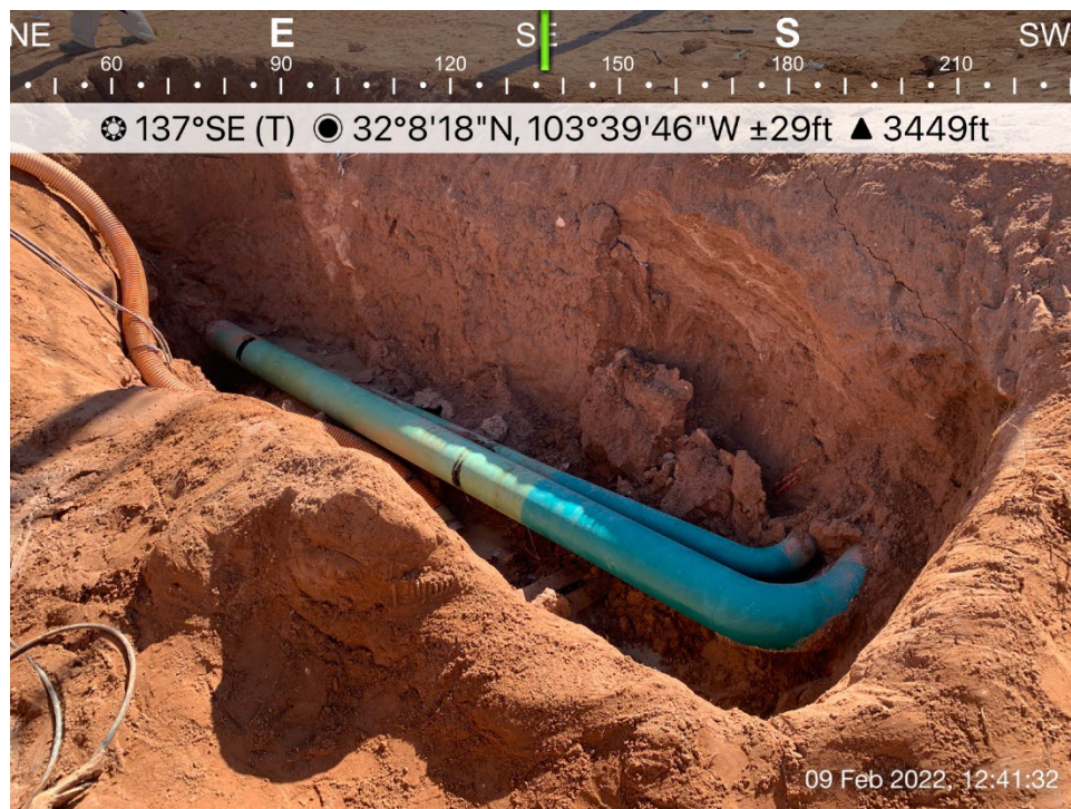
View of impacted line, February 9, 2022
