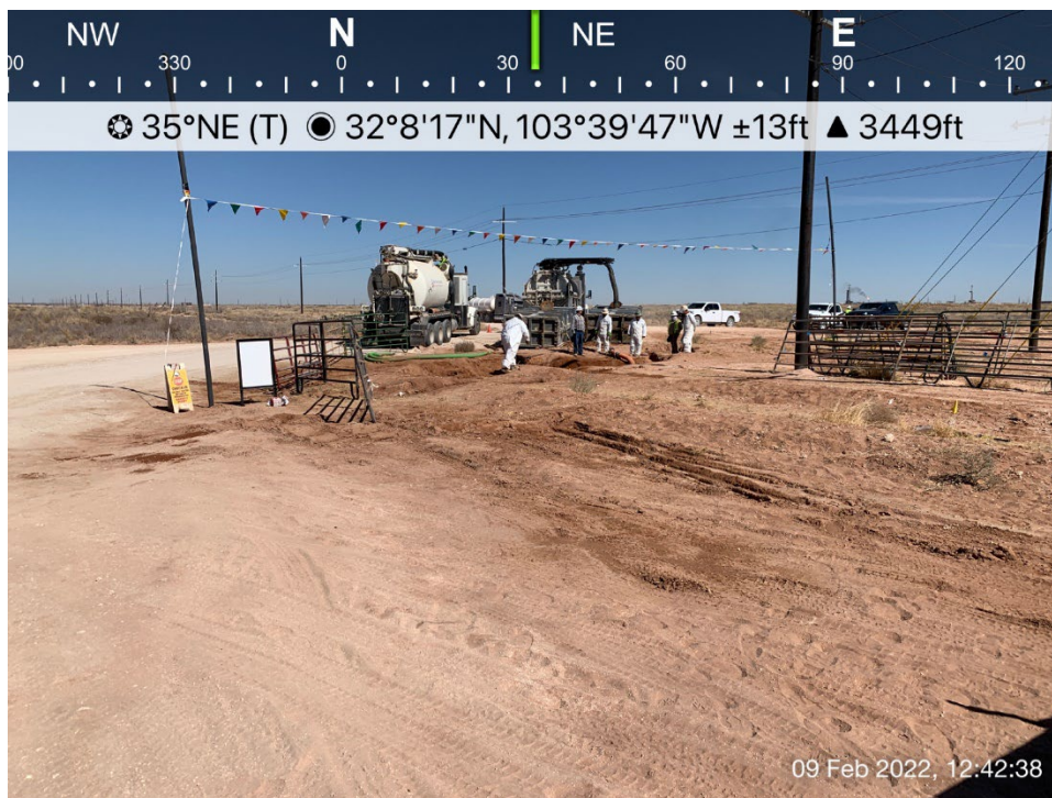
Impacted area viewing northeast, February 9, 2022
