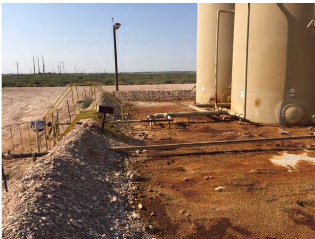
NEL 4 SWD Battery - Release (Looking South)
