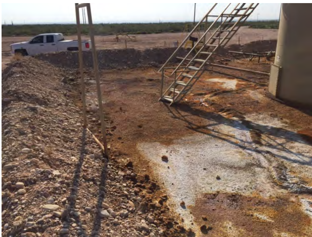
NEL 4 SWD Battery – Release (Looking East-Southeast)
