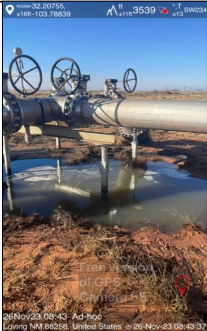
Photograph: 1 Date: 11/26/2023 Description: Produced water in release footprint View: Southwest
