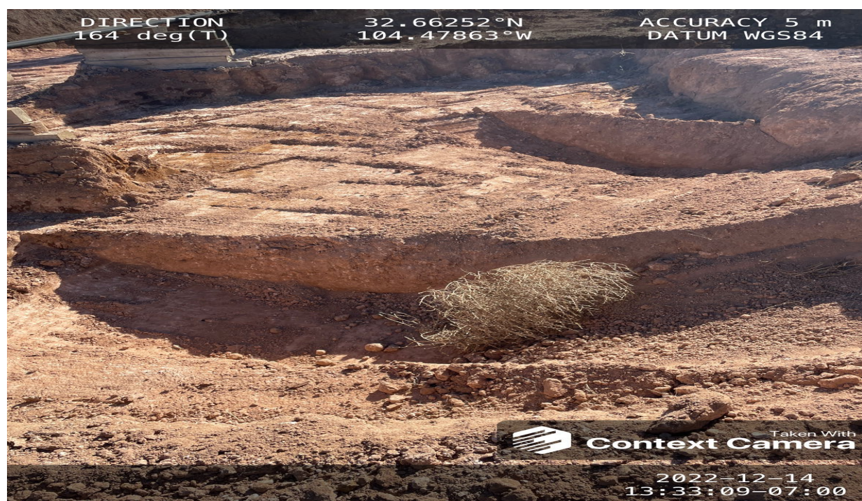
PHOTO 12: View of potholed Center area.
