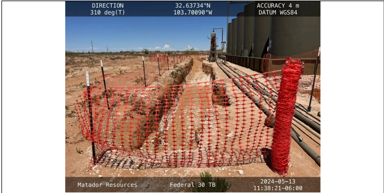
Photograph No. 3 Description: View of excavation on southwest side of tank battery
