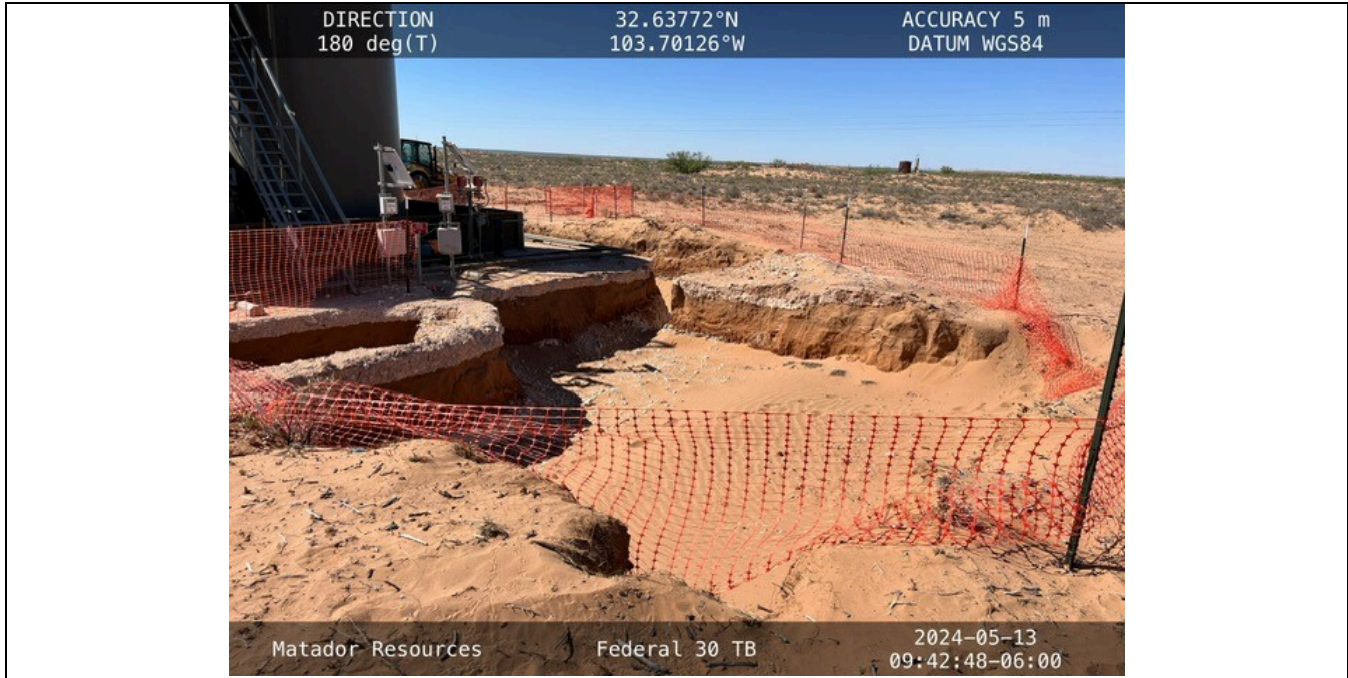
Photograph No. 5 Description: View of excavation on northwest side of tank battery
