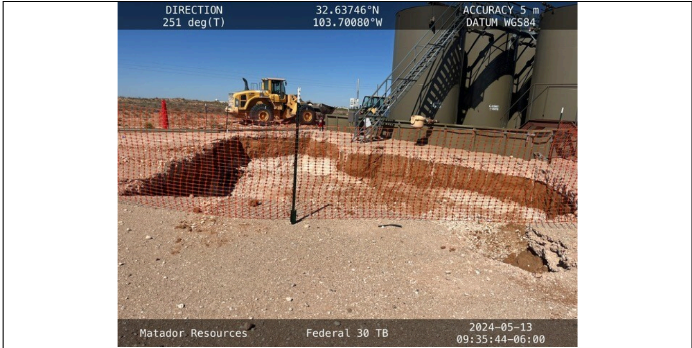
Photograph No. 1 Description: View of excavation on southeast side of tank battery
