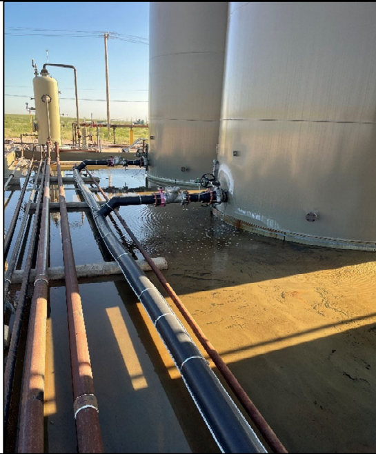
Photograph: 1 Date: 8/7/2024 Description: Free standing fluids inside containment View: South
