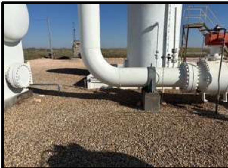
Photo of Purge Point facing North
