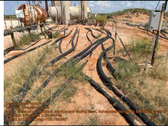
West of production equipment facing east. Advanced borehole BH25-22 west of BH25-09.
