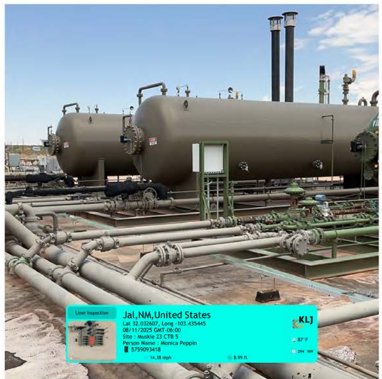
View of liner facing northwest towards equipment.
