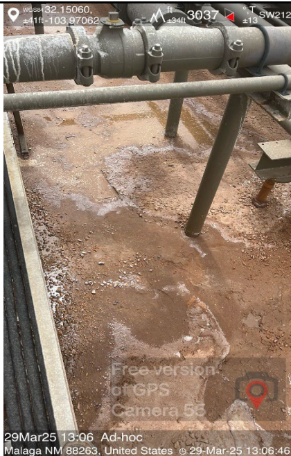
Photograph: 3 Date: 3/29/2025 Description: Initial release out of containment View: Direct
