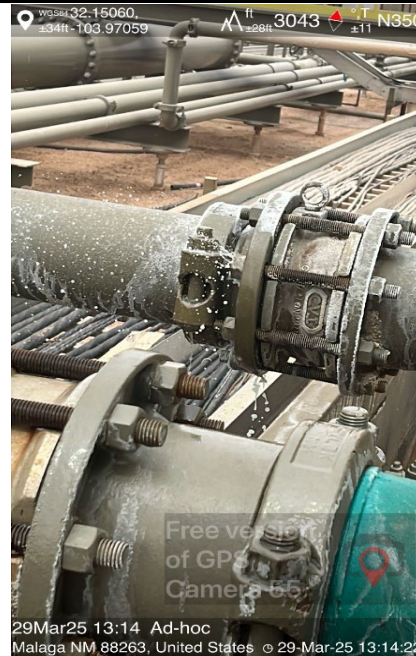
Photograph: 2 Date: 3/29/2025 Description: Initial point of release View: North
