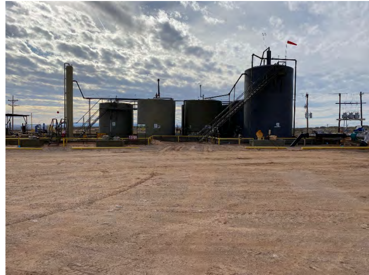
Photograph 2: View of pad and SWD tank battery – looking west
