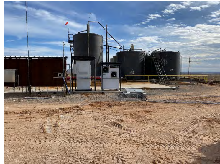
Photograph 4: View of pad and SWD tank battery – looking south.
