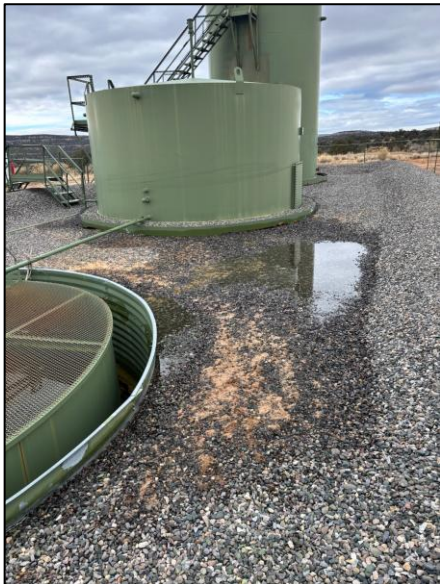
Photograph: 1 Date: 01/07/2025 Description: Soil Staining and Oil in Release Footprint View: Northwest
