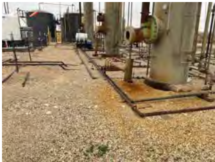
Photograph 3: Surficial staining between equipment.
