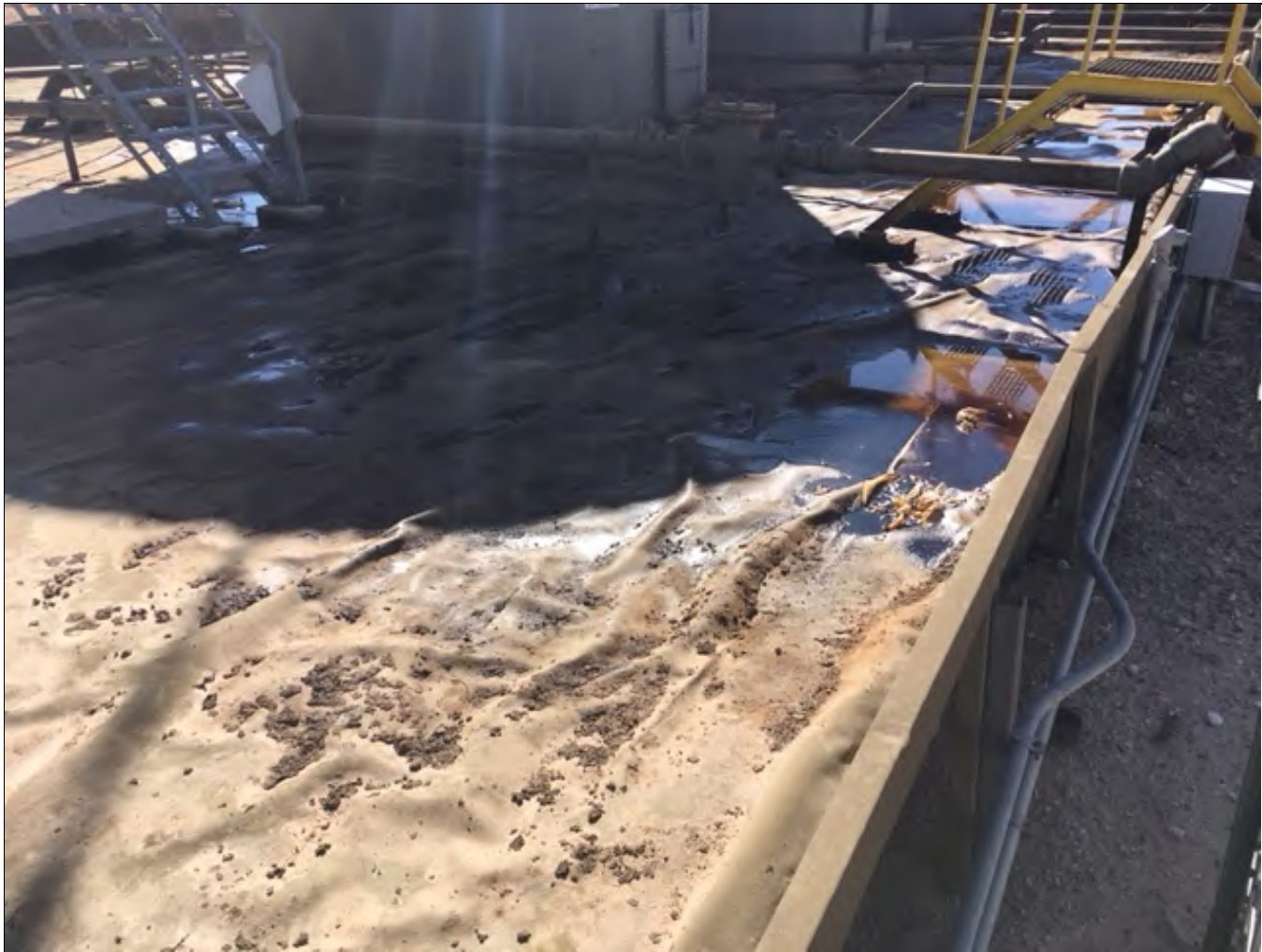
View of lined tank battery containment and liner hole during soil sampling activities.
