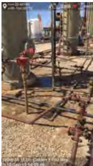
Photograph 1: Northwest view of release staining between equipment.
