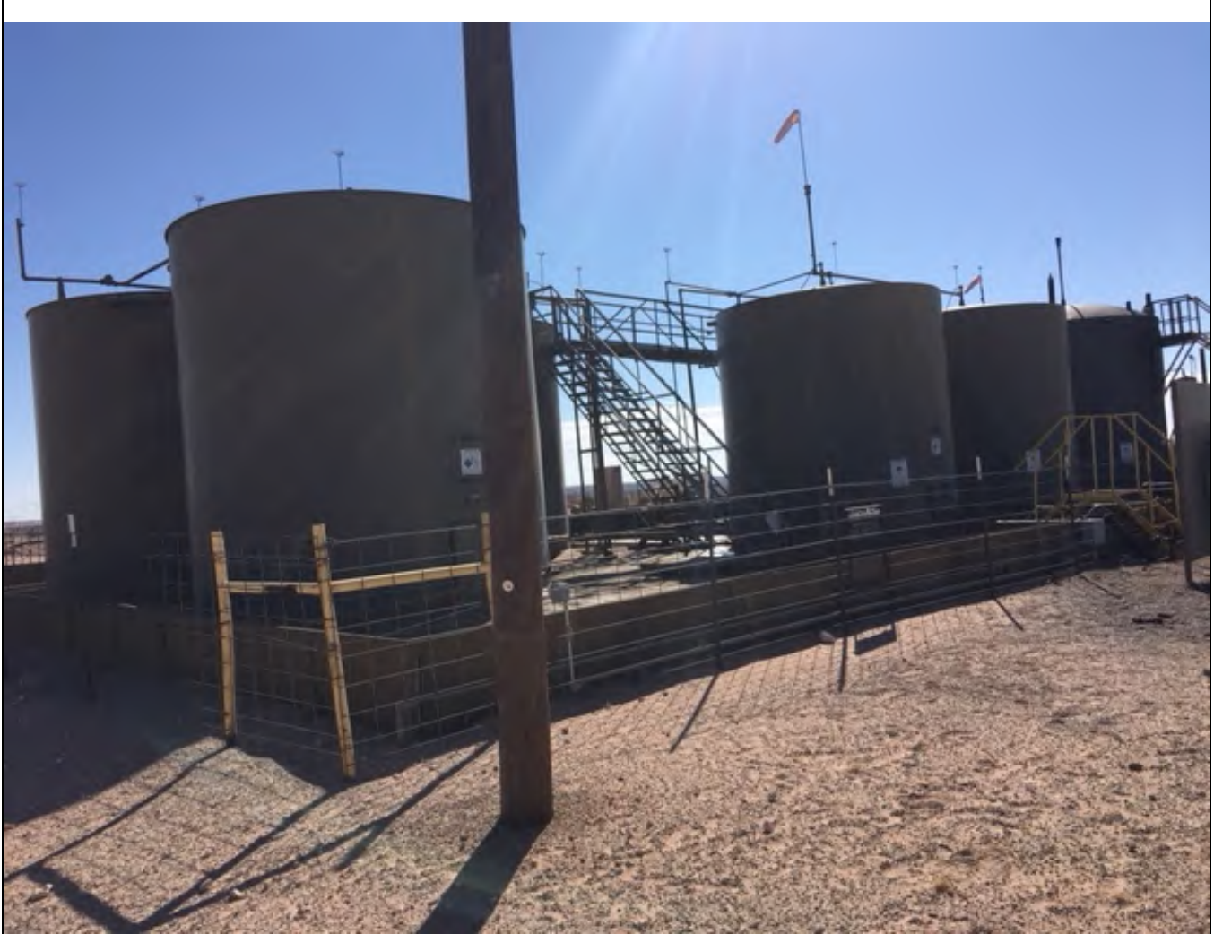
Western view of lined tank battery containment.
