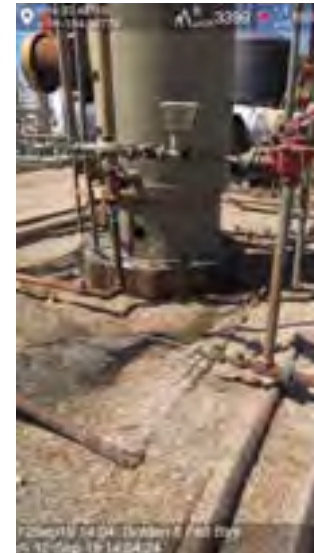
Photograph 8: Surficial staining before hand shoveling activities.
