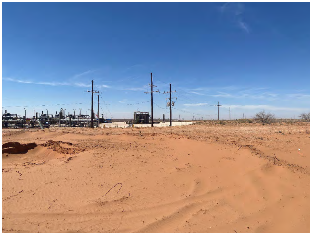
Photograph 6 (03/05/2025): Central western portion of excavation where CS-6 is located at 1' bgs. CS-8 sample location is shown to the left of the photograph at 4' bgs; facing south.
