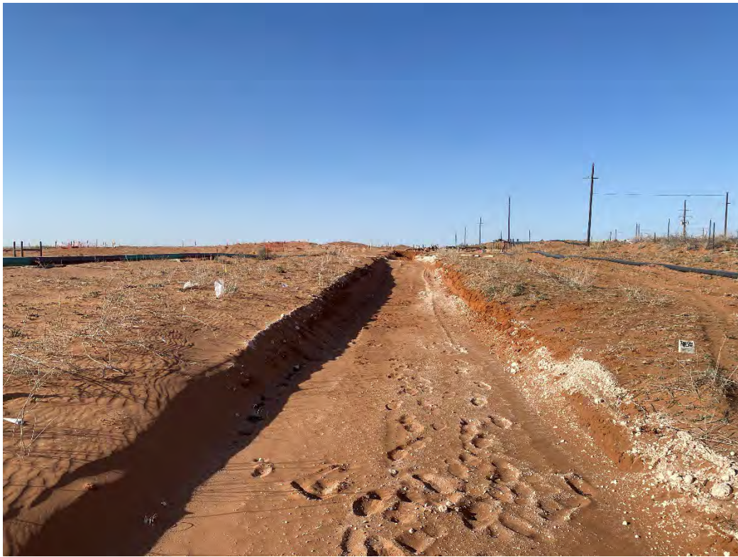
Photograph 19 (03/12/2025): Central southern portion of excavation where CS-61 through CS-66 samples are located at 2' bgs with no caliche road; facing north.
