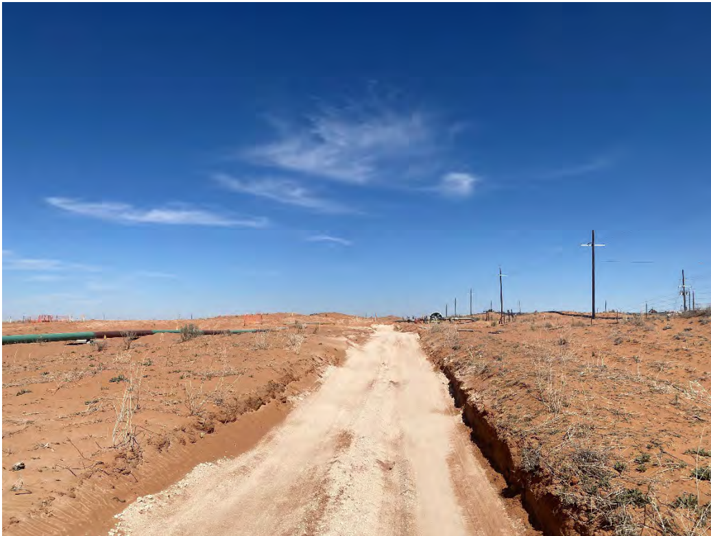
Photograph 9 (03/07/2025): Central southern portion of excavation where CS-61 through CS-66 samples are located at 2' bgs. Caliche road for hydro-excavation truck; facing north.
