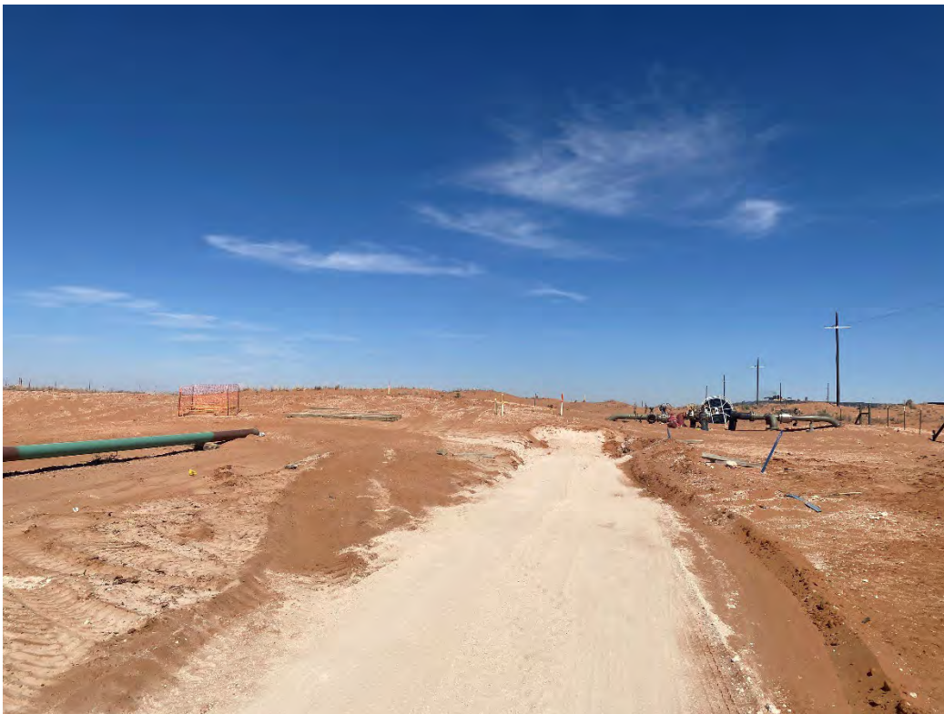
Photograph 10 (03/07/2025): Central northern portion of excavation where CS-51 is located at 1' bgs; facing north.
