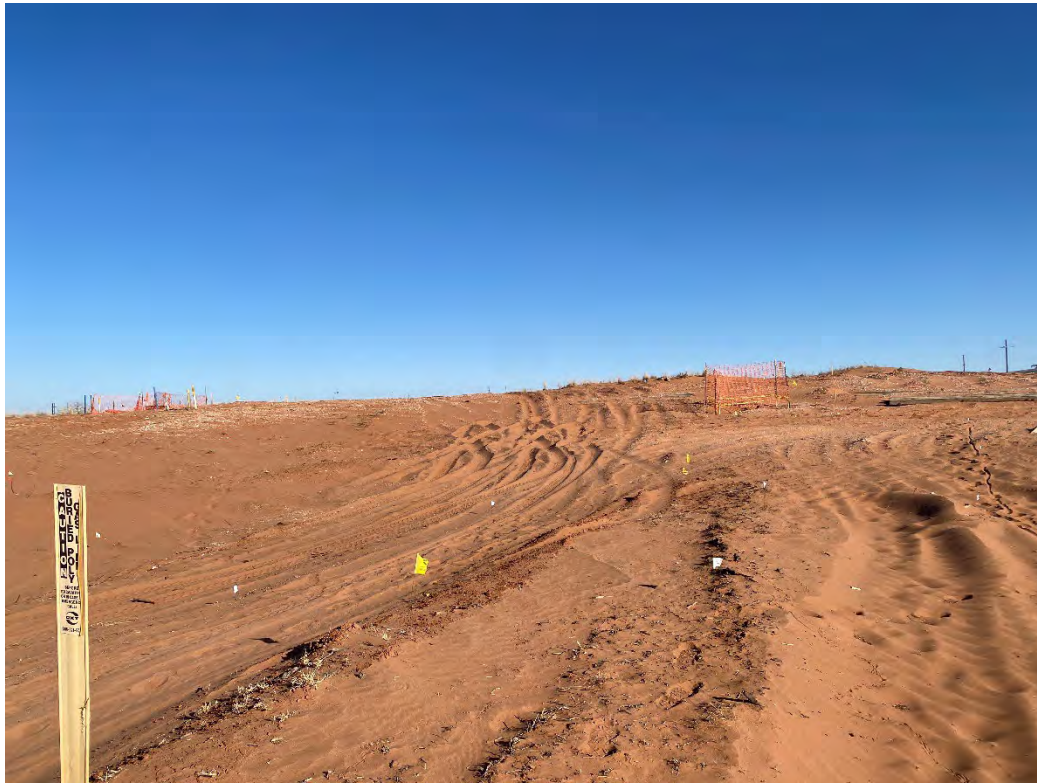
Photograph 11 (03/07/2025): Standing at sample location CS-32 while overlooking confirmation sample flags in the central northern portion of excavation at 1'bgs; facing north.
