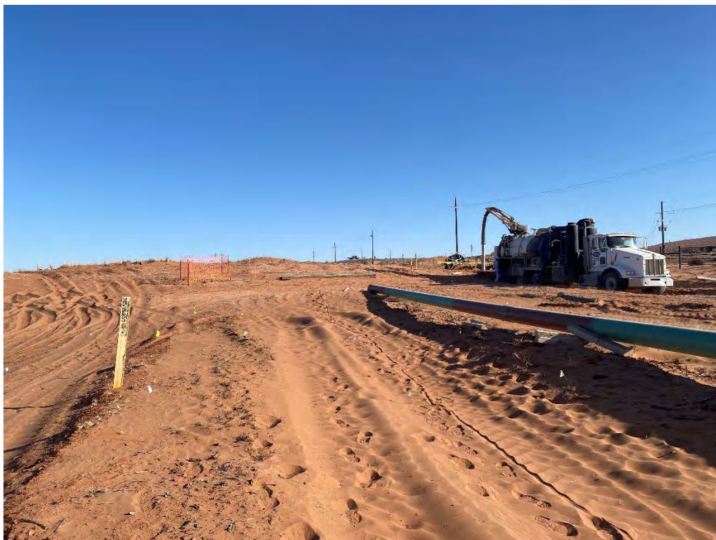
Photograph 12 (03/07/2025): Standing at sample location CS-32 while overlooking confirmation sample flags, aboveground pipeline, and hydro-excavation truck; facing northeast.
