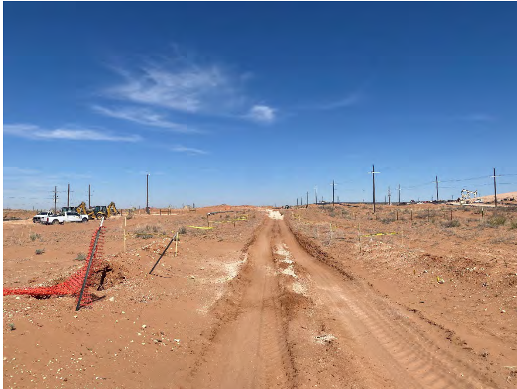
Photograph 5 (03/05/2025): Southern portion of impacted area at 1' bgs at CS-74; facing north.
