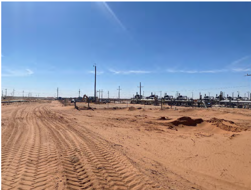
Photograph 7 (03/05/2025): Central western portion of excavation where CS-21 sample is located; facing southwest.
