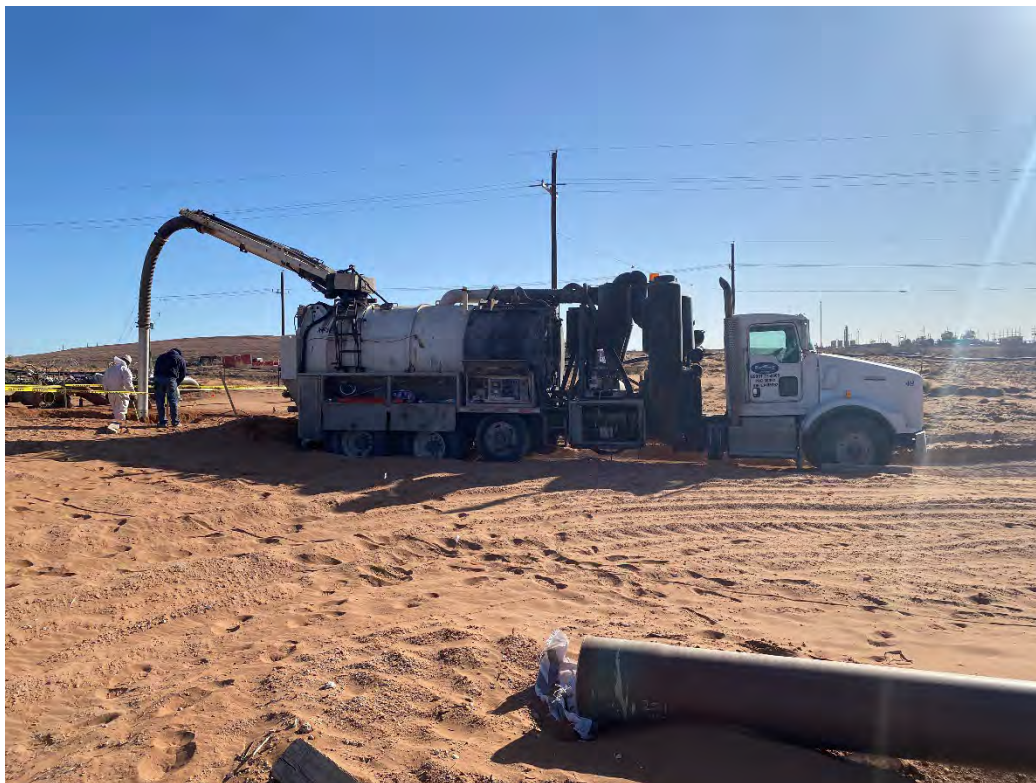
Photograph 14 (03/07/2025): Standing at sample location CS-31 overlooking hydro-excavation truck working on sample location CS-53; facing east.
