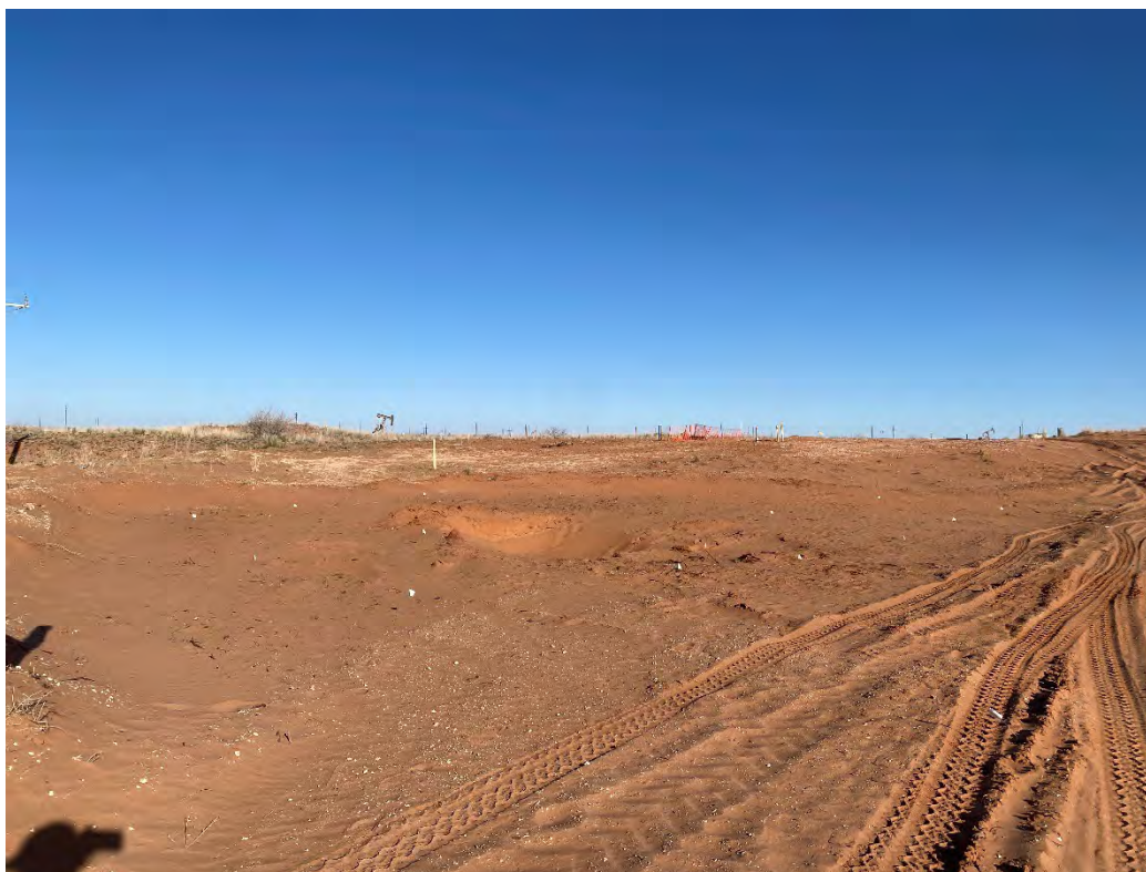
Photograph 8 (03/07/2025): Central western portion of excavation where CS-21 sample is located. Sample flags have been marked for confirmation sampling; facing northwest.
