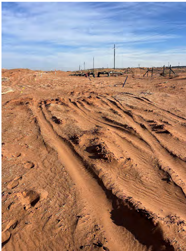
Photograph 2 (02/19/2025): Central northern section of the delineated area prior to excavation. Lay flat produced water pipelines shown; facing north.
