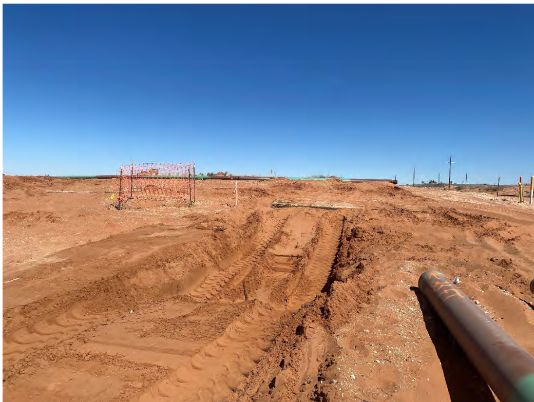
Photograph 21 (03/24/2025): Additional excavation at sample location CS-21 and CS-30 to 4' bgs; facing north.
