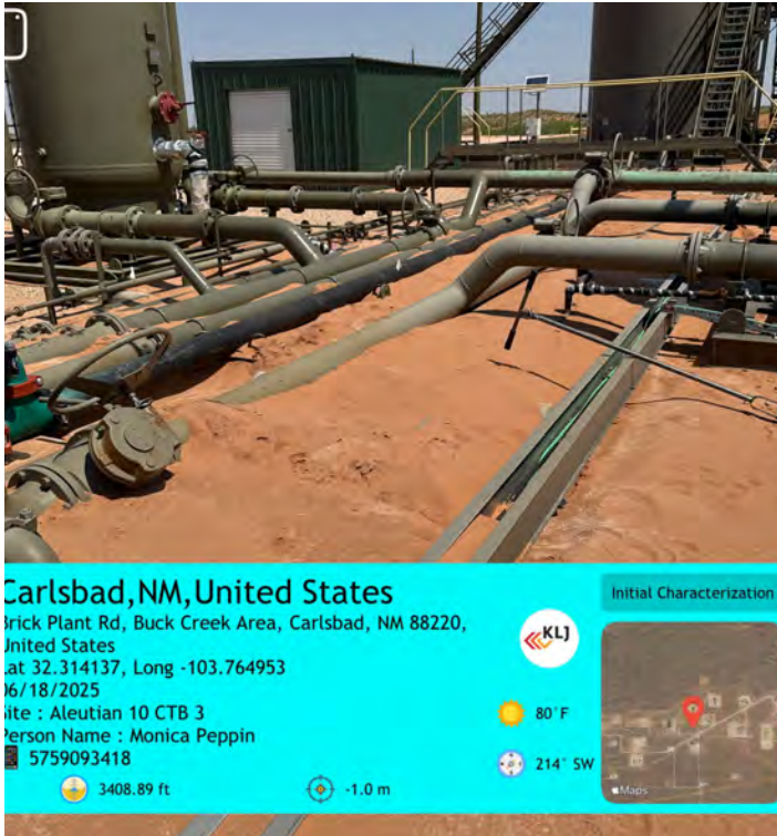
Release area under piping near point of release and BH01.
