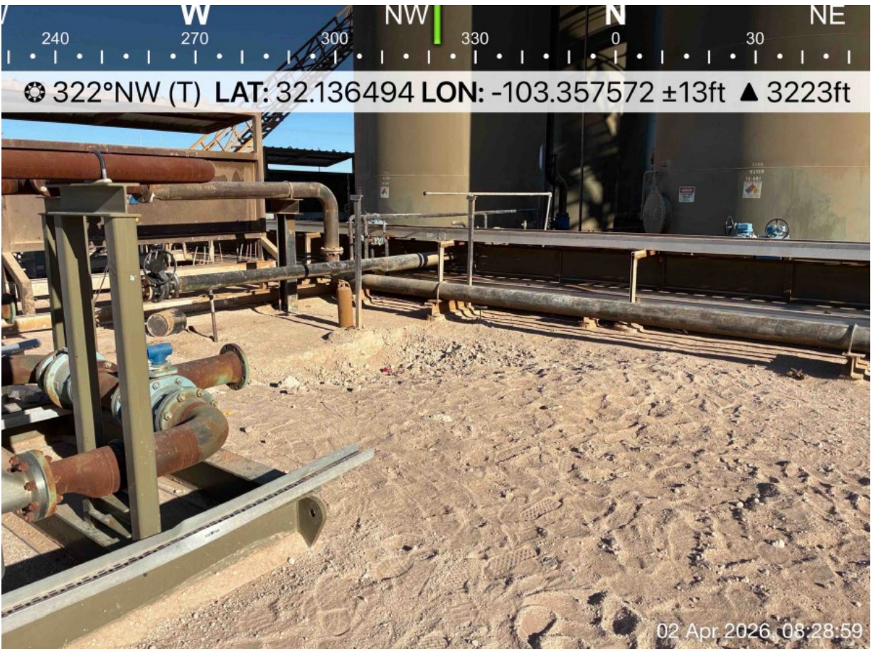
4/2 - shows the addition of the 2nd pumping unit
